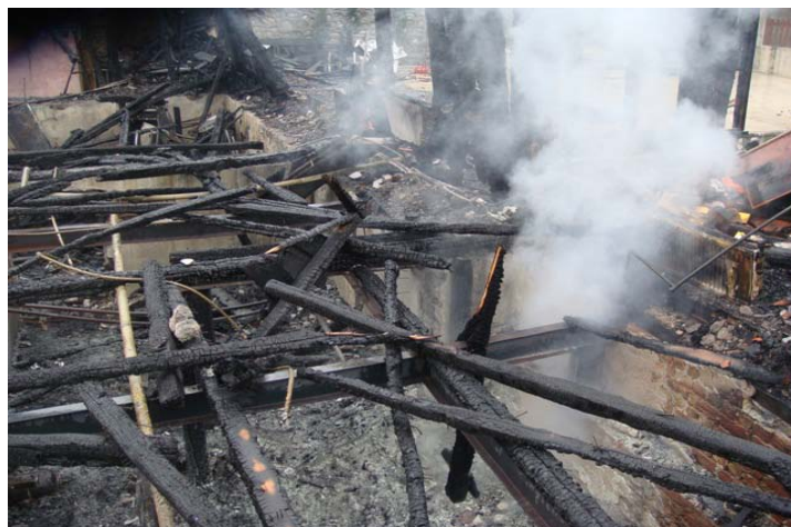
Figure 5 Selami efendi Tekke, the situation of timber structure after fire [11]
