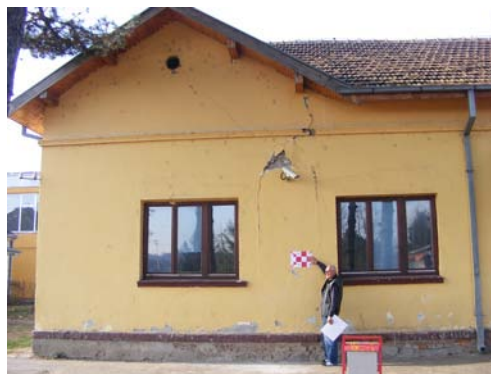
Figure 23Figure 20. Characteristic Damages
