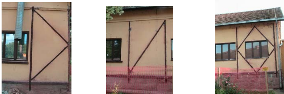
Figure 27. Wall prepared for installation of vertical stiffeners type, “D”, “R” and “K”
