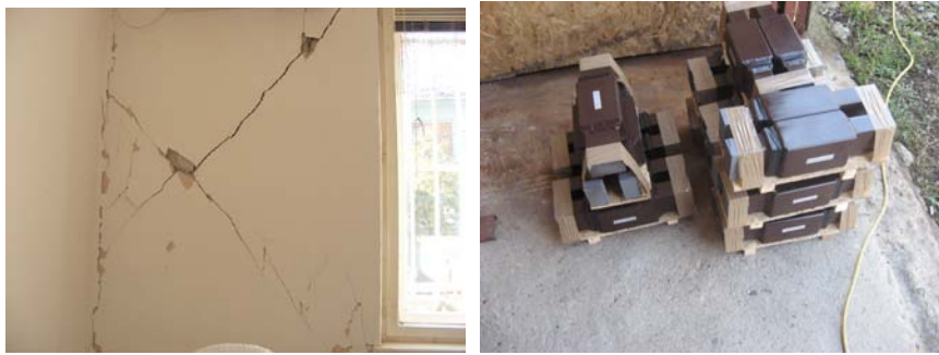
Figure 7. Characteristic Damages, X cracks, and Dampers
