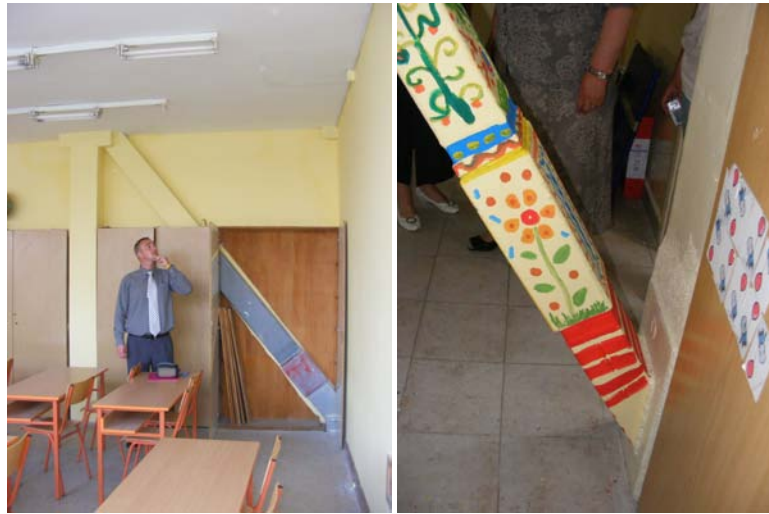
Figure 5. Vertical stiffening in longitudinal Y-direction diagonal square cross-section 260x160x7 with damper. Force in damper +- 1100 kN, displacement +-5mm.
