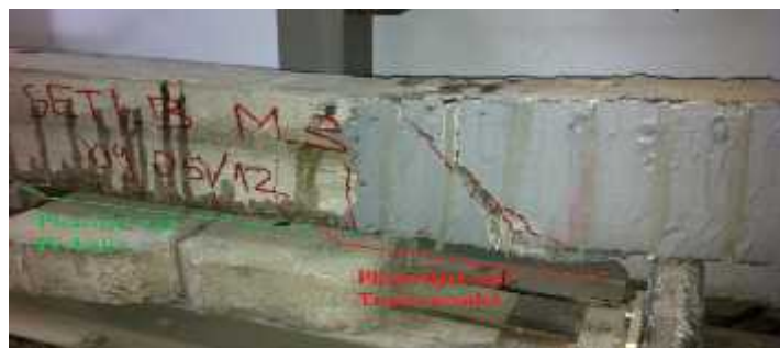
Fig.5.4. Cracks in set B/beam 3
