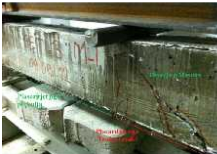
Fig.5.3- The cracks in Set B/beam 1
