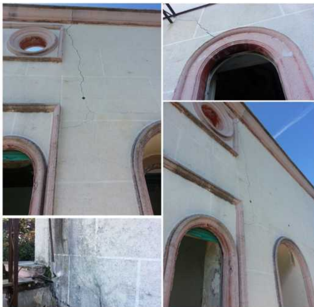
Figure 4. Cracks due to settlements
