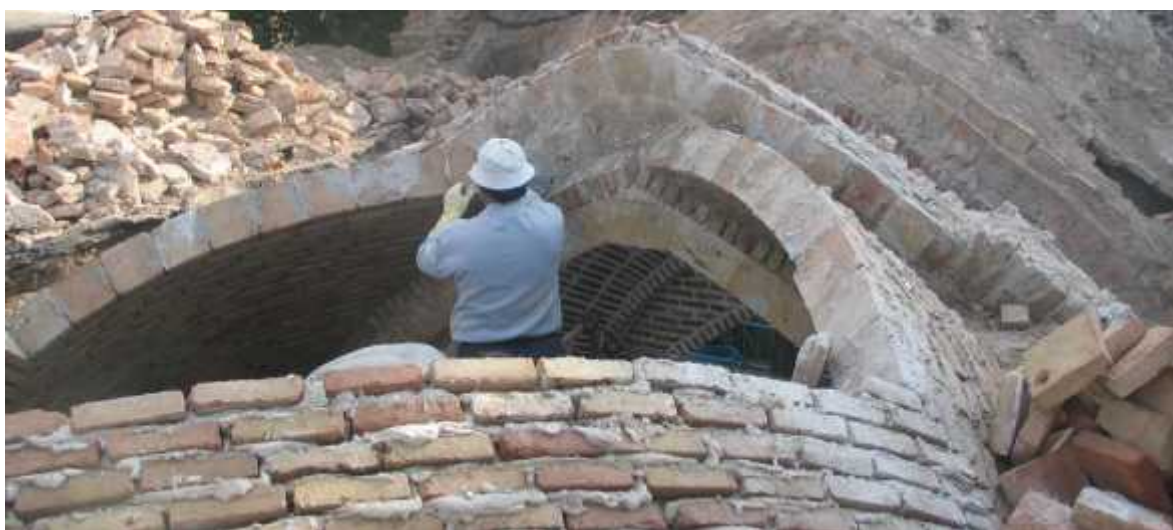
Figure 1. Restoration site inside the Bazaar of Tabriz. The picture is showing the creation of a vault without centering and the disposition of the squared bricks.
