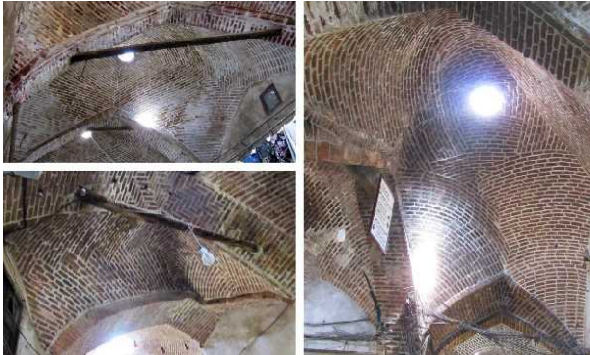
Figure 2. Pictures of the bazaar of Tabriz showing the irregular disposition of the bricks inside vaults realized without the help of the centering.
