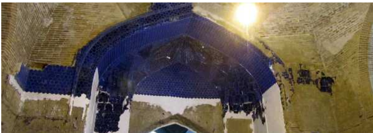
Figure 4. Masjed Kabud, Tabriz. Picture showing a decoration with little muqarnas in the corners, realized with tiles and chalk. The absence of the tiles is showing the shape of the structural part made up by bricks.
