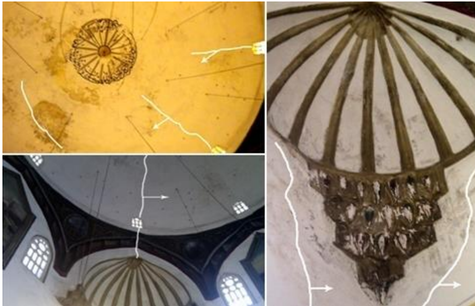
Figure 2. Cracks in the interior of the dome and pendentives in Mirahor Ilyas Beg Mosque
