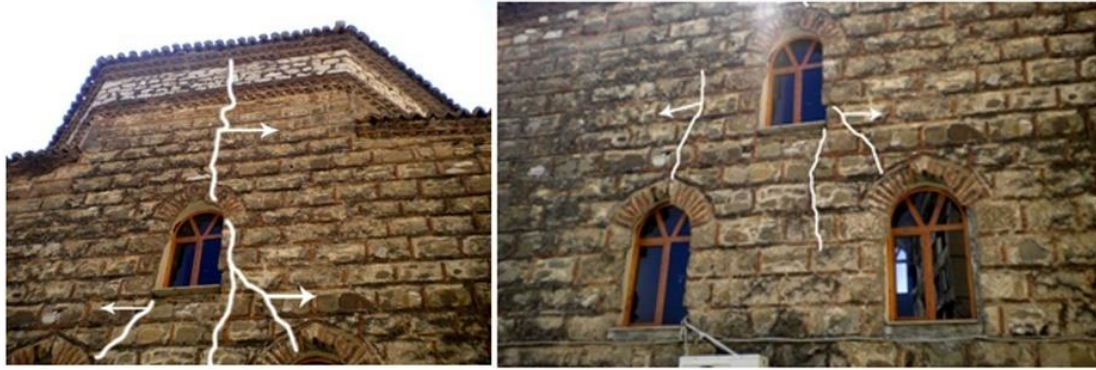
Figure 3. Propagation of cracks in the load bearing walls, west façade of Naziresha's Mosque
