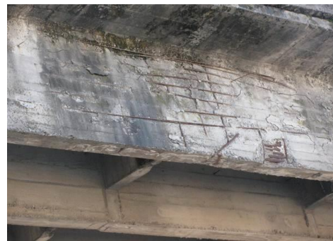
Figure 7. Spall of concrete.
