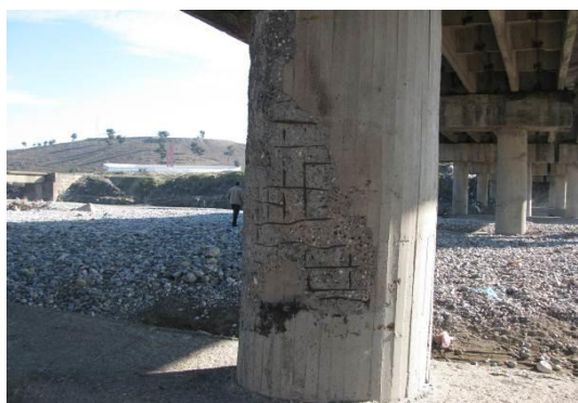
Figure 9. Damage of the column
