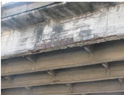
Figure 6. Spall of concrete
