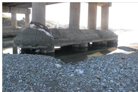
Figure 10. Damage of the piles
