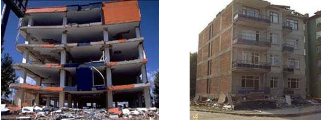
Figure 2 Reinforced concrete frame structure with embeded beams into the slab, after earthquake Gölcük, Turkey.
