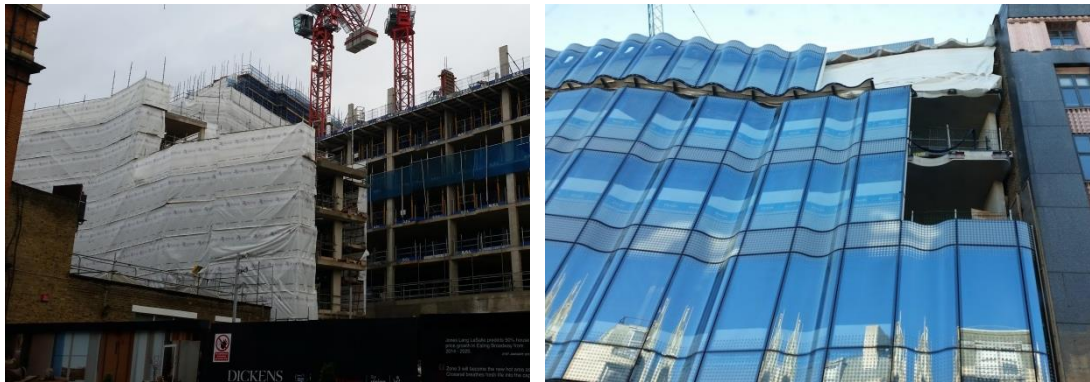
Figure 2. Comparison of stick and unitized facade constructions (a stick curtain wall, left, requires scaffolding and is labour intensive on site; unitized curtain walls, right, minimise the safety hazards on site due to the reduced field handling).
