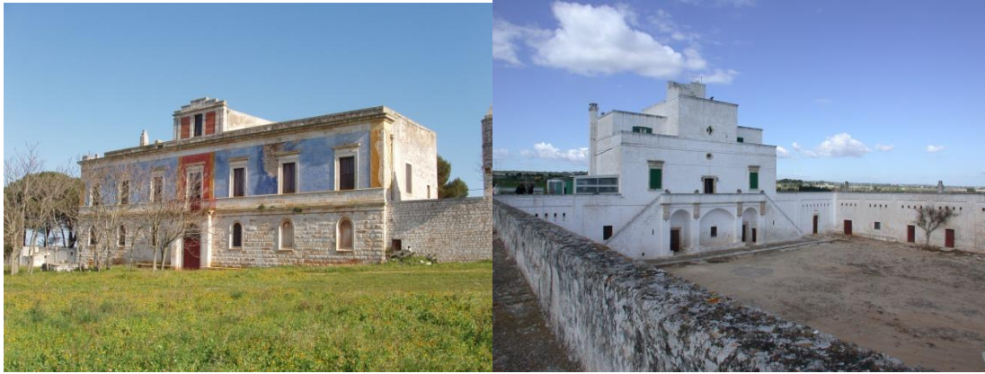
5. Openings and main facades Masseria Santissimo – Turi (Ba). 6. Internal courtyard Masseria Miani – Polignano (Ba).
