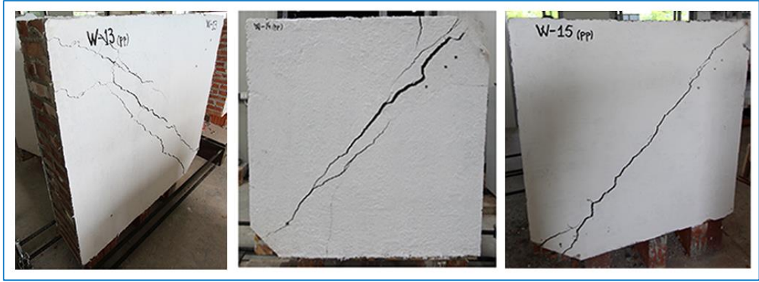
Figure 33. Failure mode of polypropylene reinforced mortar strengthened wall panels of Series 1.
