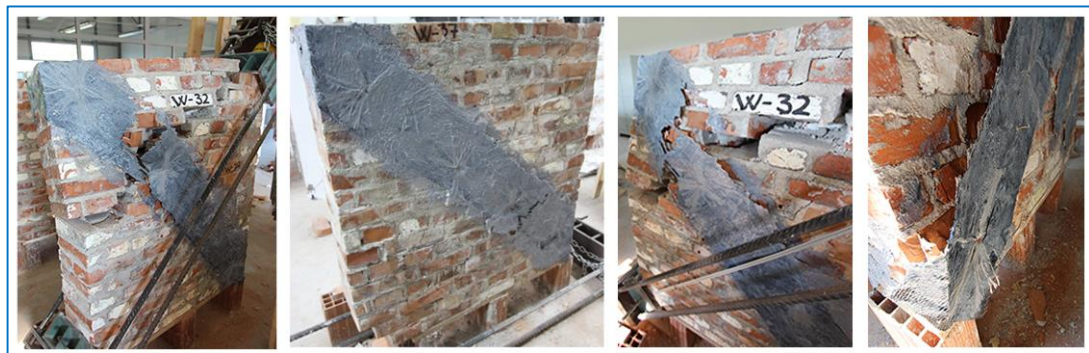
Figure 36. Failure mode of C-FRP strengthened wall panels of Series 2.
