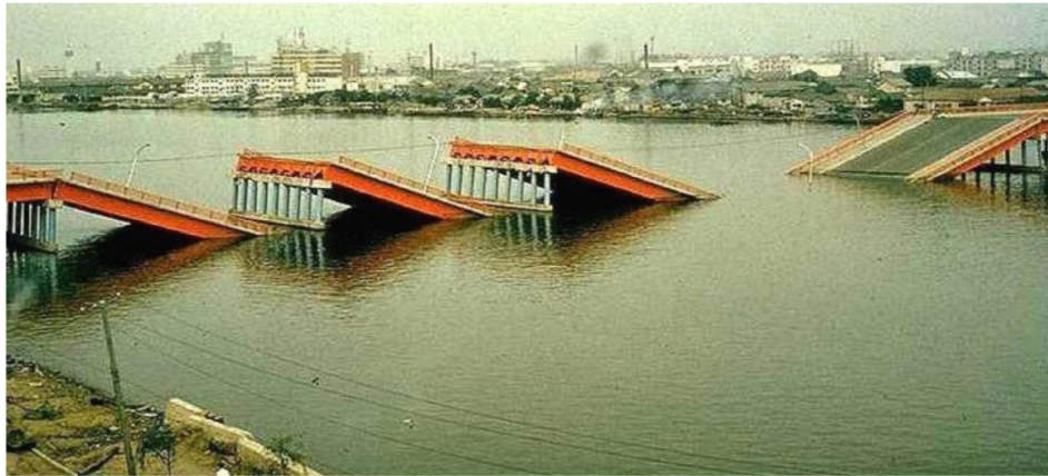
Figure 5. The destruction of the bridge as the result of lateral spread, Niigata 1964 [5]
