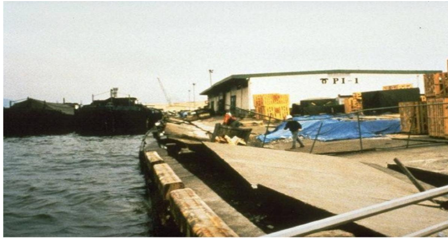
Figure 3. Damages seen in Kobe port in Japan during the earthquake of 1995 due to the occurrence of the phenomenon of liquefaction [3]
