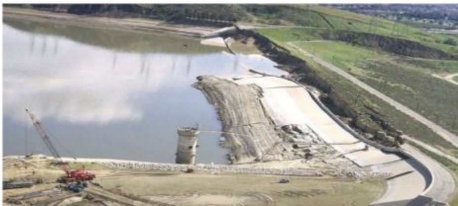
Figure 2. Huge damages on the dam's wall happen due to the lateral spread, Kobe 1995 [2]
