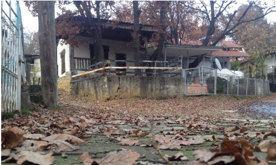
Figure 29. Nashec: House in poor condition
