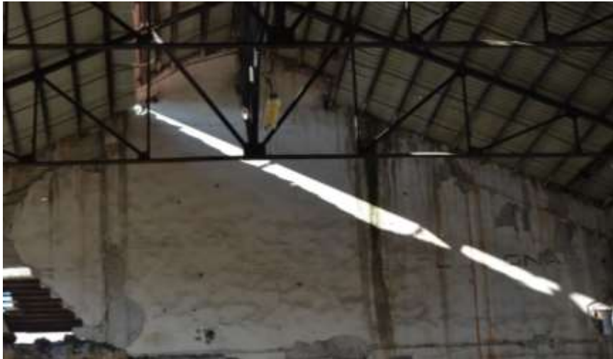
Figure 132. Photo of the inner wall at the ex-TEC, Kuçova [ elaborated by the author ]
