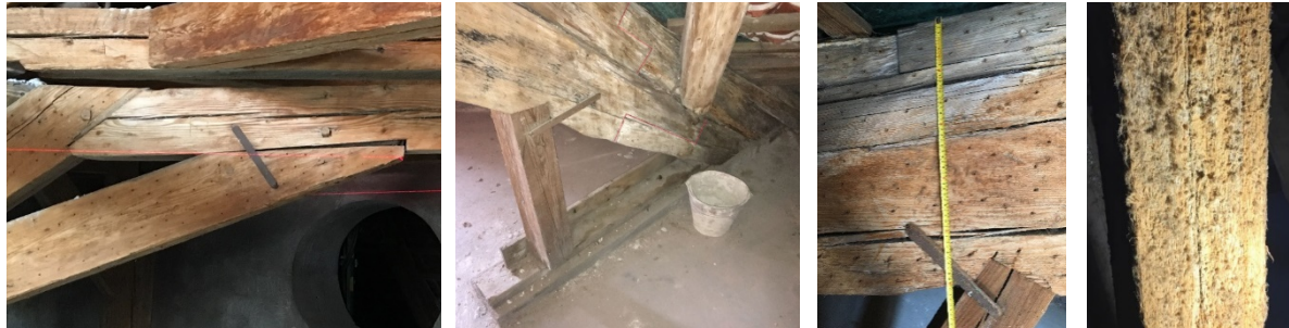
Figure 4. Characteristic features on the elements from the visual inspection;
