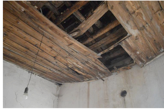
Figure 4. Presence of Humidity and degradation of wooden ceiling
