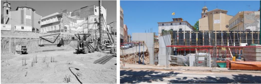
Figure 4: Retaining wall constructed by piles and early stages of the new Hall.
