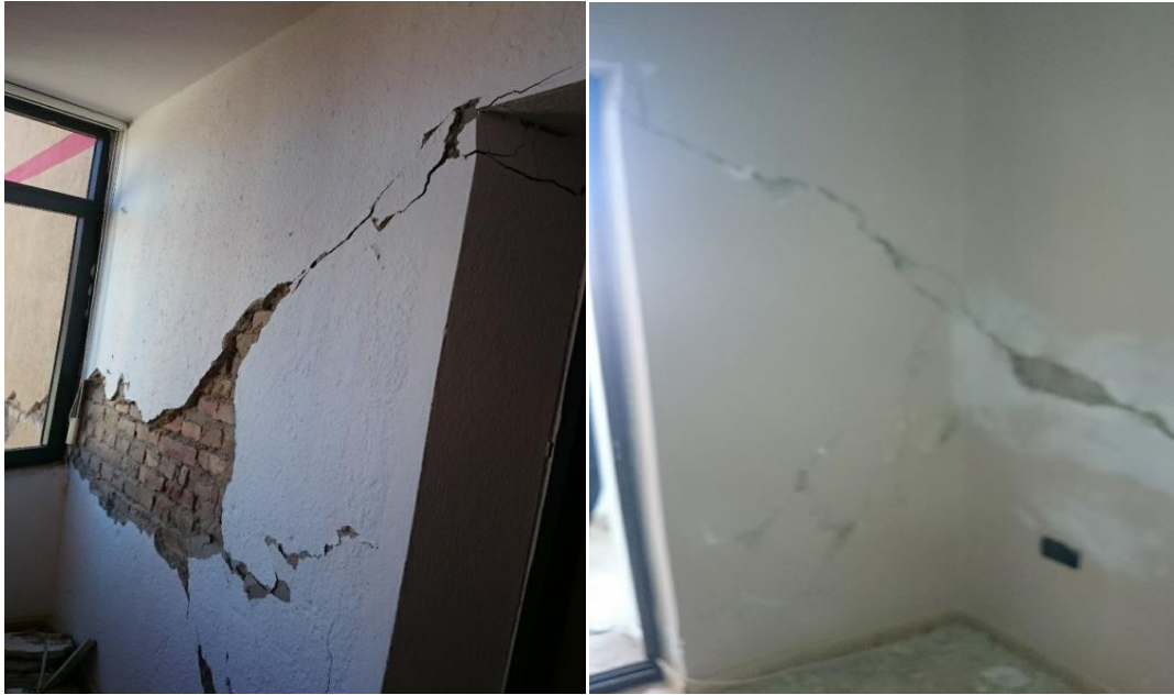
Figure 270: Heavy shear cracks on load bearing walls on the second floor
