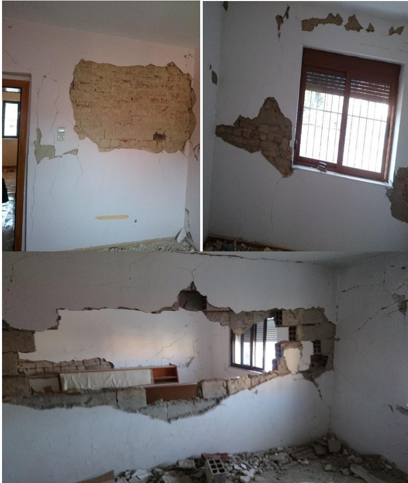
Figure 267: Typical damage patterns observed at several locations of the building block 11/1. As seen from the photos, the material quality especially the mortar is very weak and could not prevent the spall of the bricks. Damage was concentrated on the 2 nd and 3 rd floors. Level of the damage on load bearing walls was moderate whereas the partition walls were heavily damaged. This building suffered not only non-structural damage but also very heavy structural damage with some separation on load bearing walls due to reasons comprising old construction age, poor quality of material and construction, poor workmanship, interventions made by people, the design code of the time- if ever was applied-lack of maintenance and inadequate repair after previous damaging seismic events. Typical damage patterns like spall of mortar and separations on the corners, spall of mortar and sprandel cracks near the window openings, partial collapse of partition walls are observed and are shown in the figures above. Shear cracks in load bearing walls are (25-30) mm wide.
