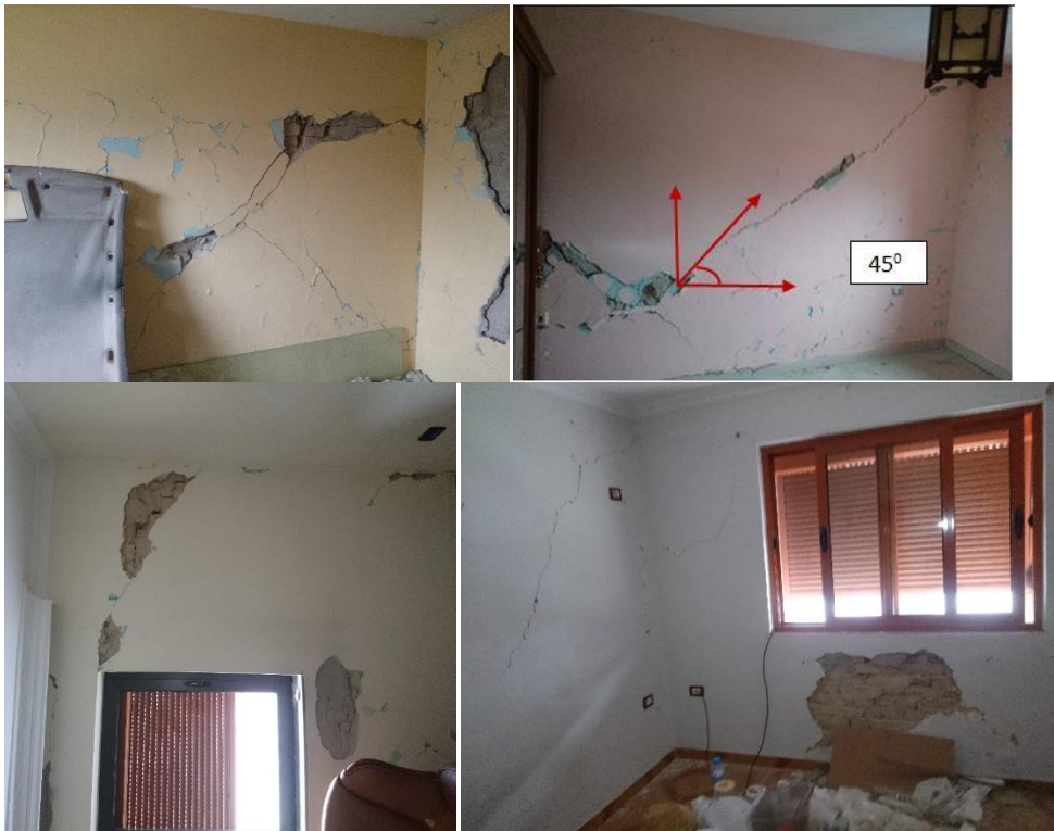
Figure 264: Typical damage patterns observed at several locations of the building nr.5 blocks
