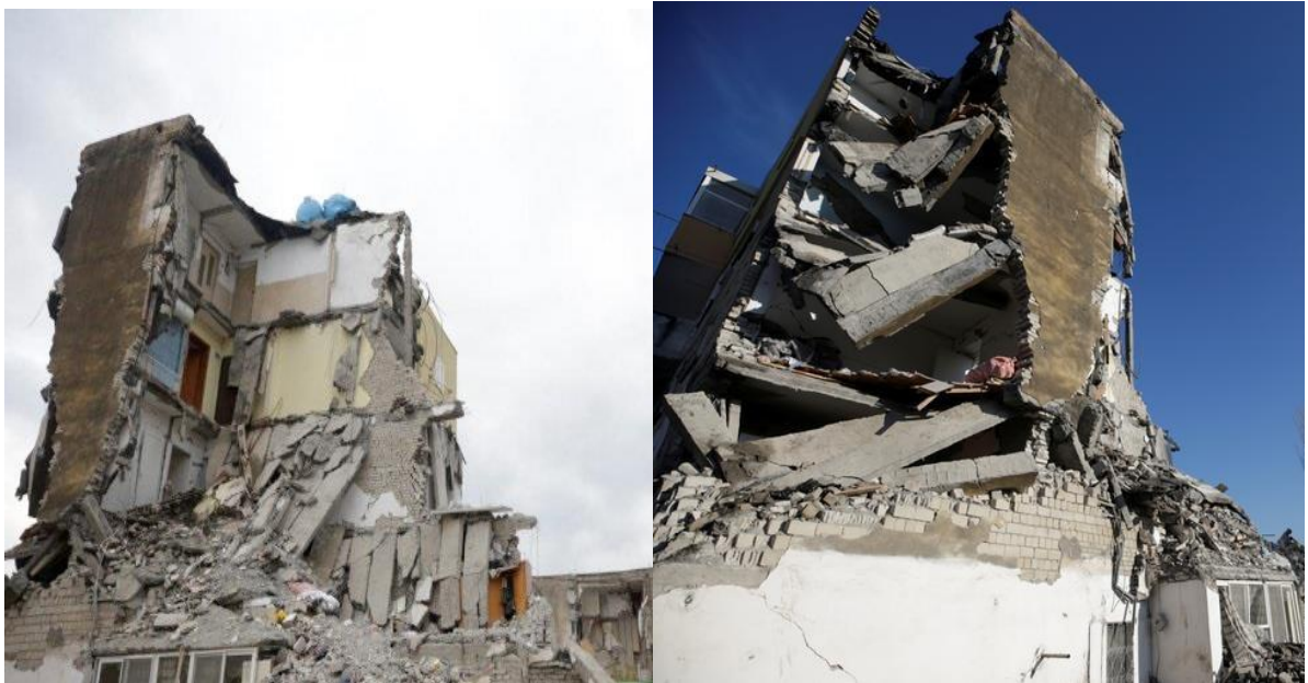
Figure 254: Collapsed masonry building in Thumane
