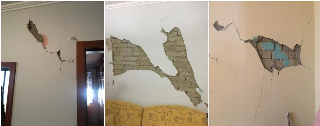
Figure 275: Light damage patterns on non-structural elements
