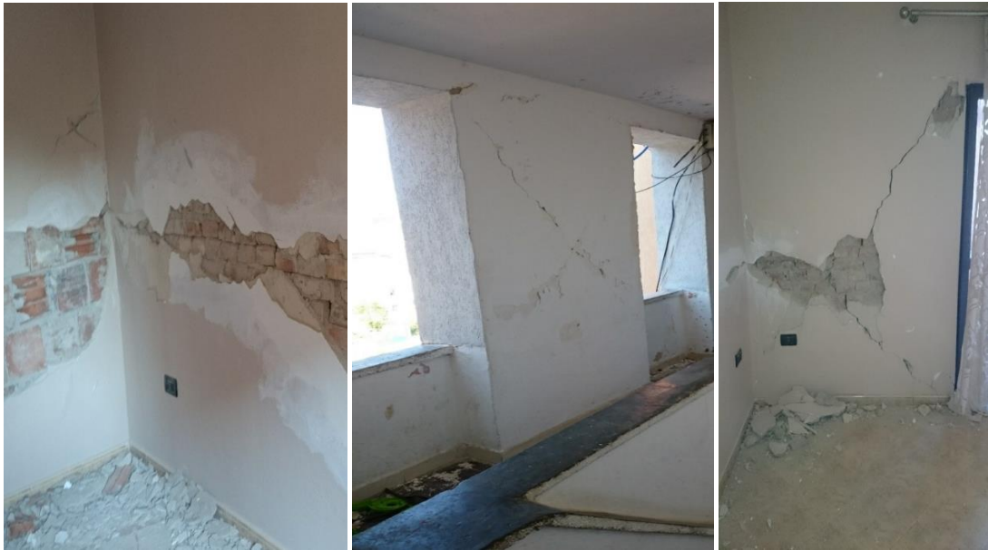
Figure 269: Serious shear cracks on load bearing walls and the piers of the building
