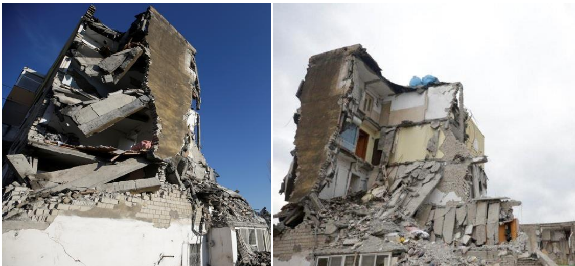
Figure 257: Collapsed building of template B2 plus one story in Thumane
