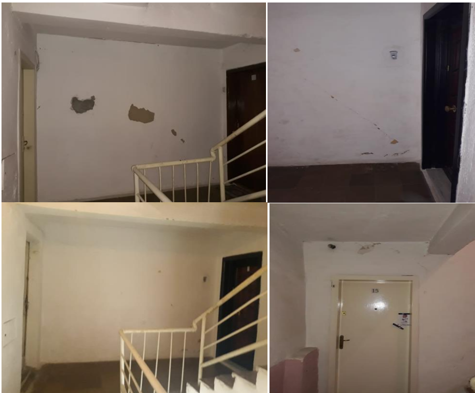
Figure 272: Light damage patterns on non-structural elements
