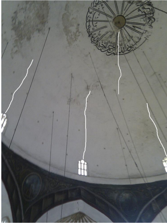
Figure 4. Cracks on the dome and spalling of plaster
