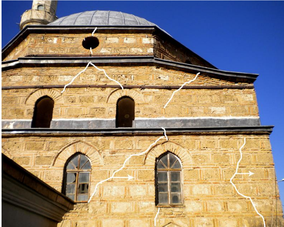
Figure 5. Cracks on the load bearing walls in the south facade of the mosque
