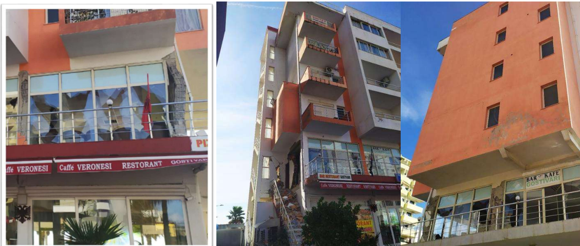
Figure 9. Damages in Buildings of more than 5 storeys with RC frame and infill walls (Gostivari Building, Durres)
