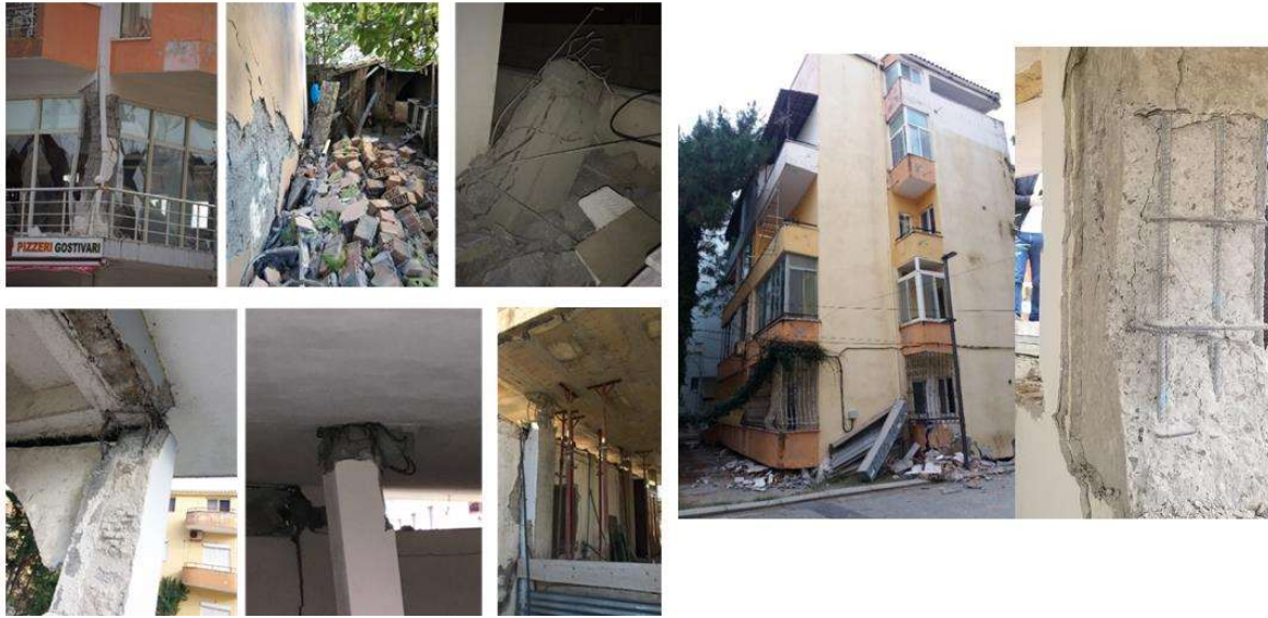
Figure 12. Problems related to poor constructive detailing
