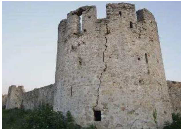
Figure 9: Existing crack of the north-eastern tower.
