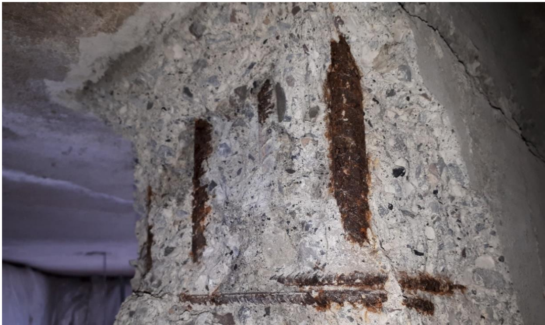
Figure 25: Corroded rebars and damaged column
