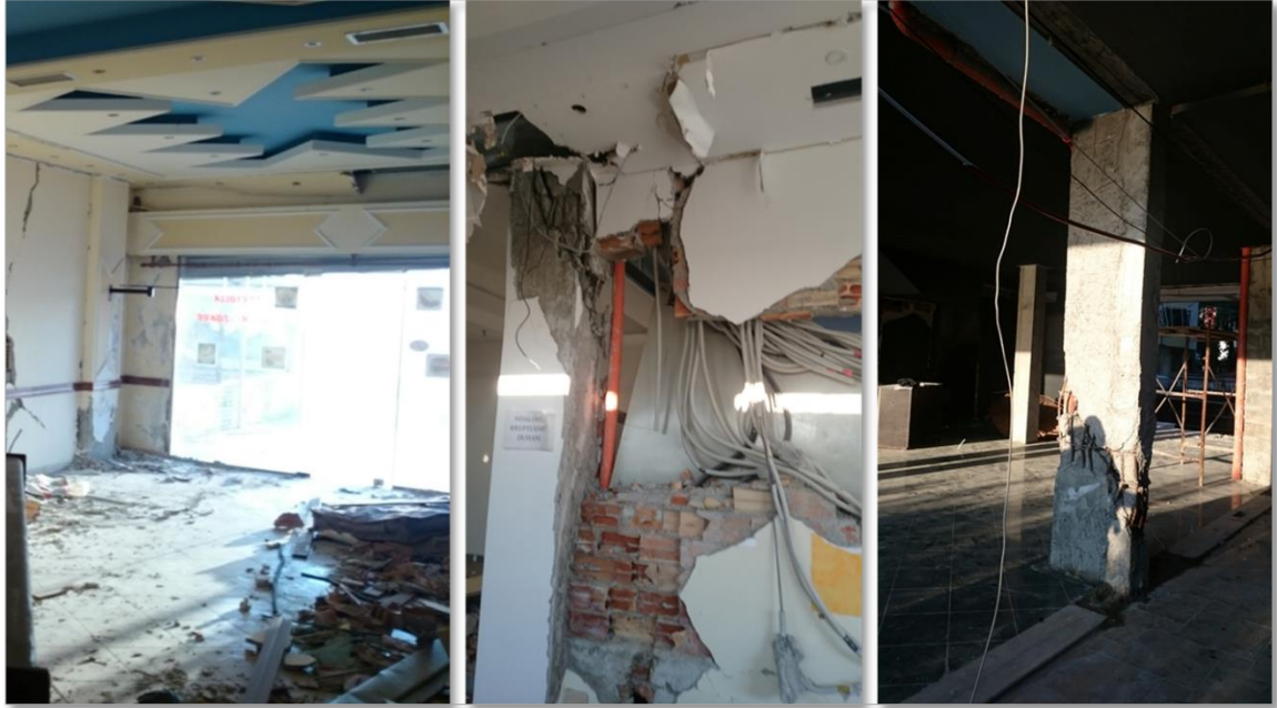
Figure 80: Damages of the E Template building during November 26, 2019 earthquake
