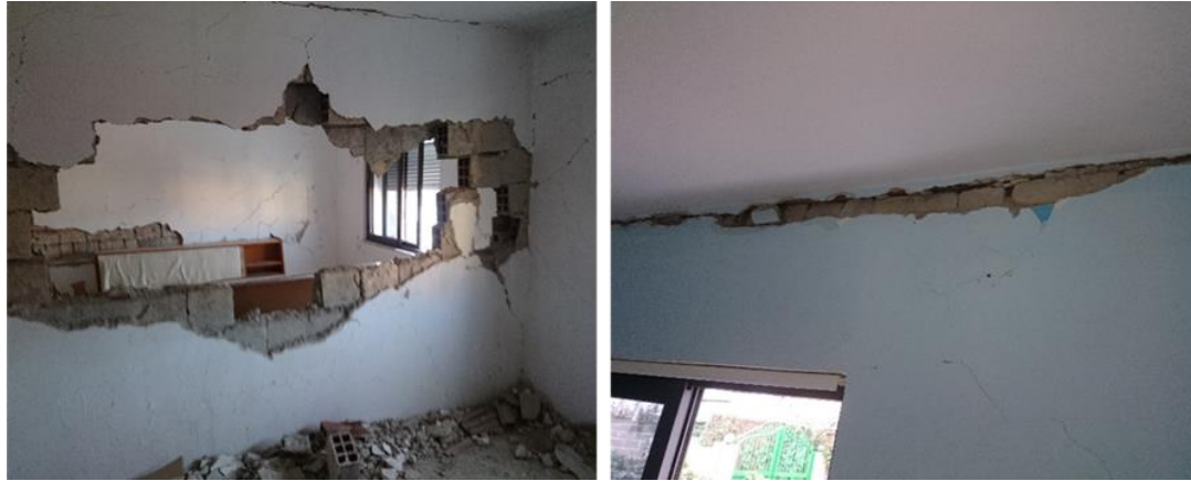
Figure 41: Out of plane failure of masonry walls
