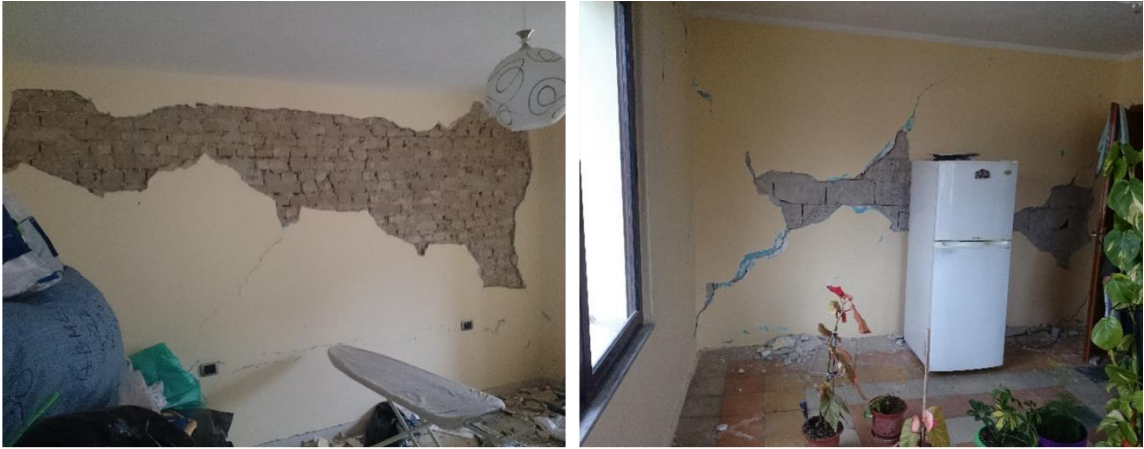
Figure 38: Spall of mortar, shear and bending cracks
