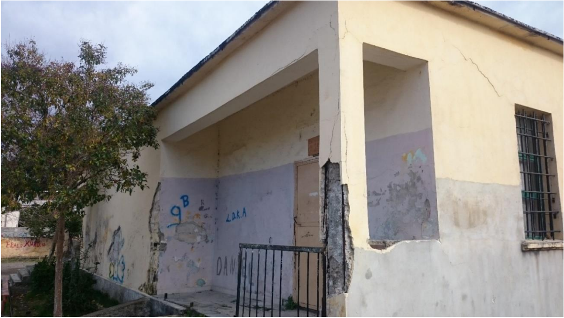
Figure 20: Reinforced concrete column with no stirrups
