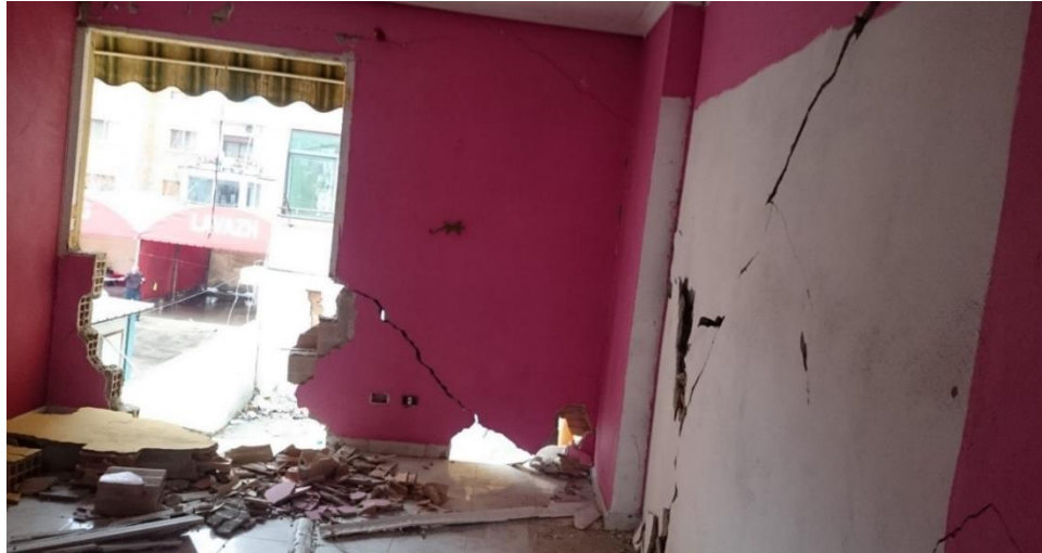
Figure 34: Out of plane failure of partition walls
