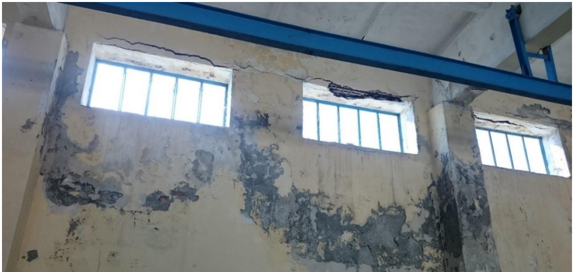
Figure 17: Short column formation and corrosion in reinforcement
