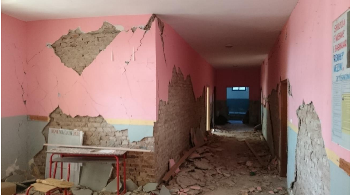
Figure 36: Heavily damaged walls on a masonry building
