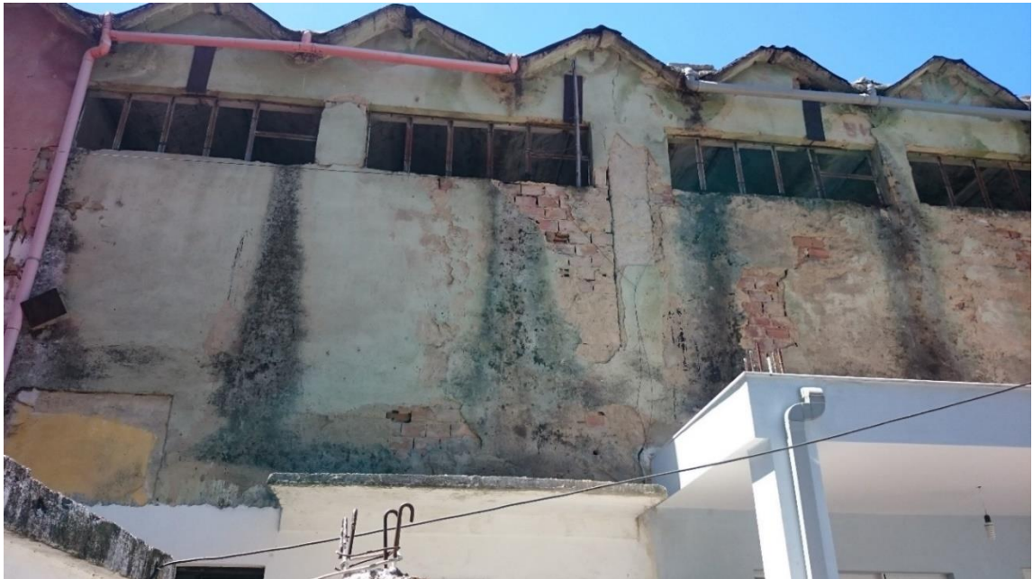
Figure 47: Damage due to short column and lack of maintenance
