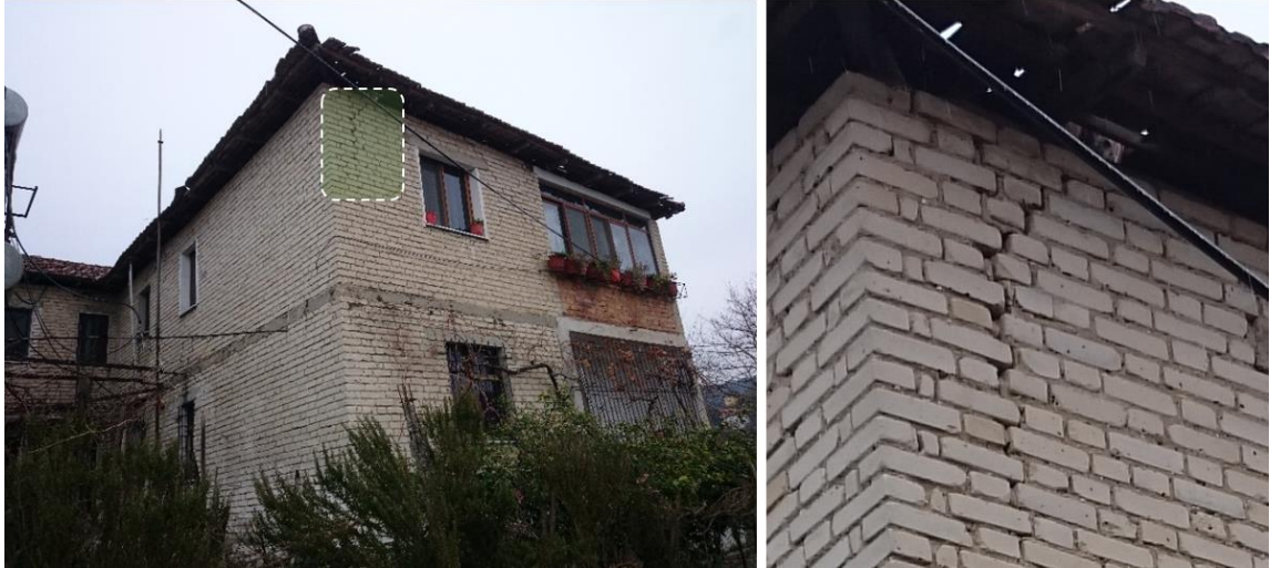
Figure 43: Observed example of return wall separation
