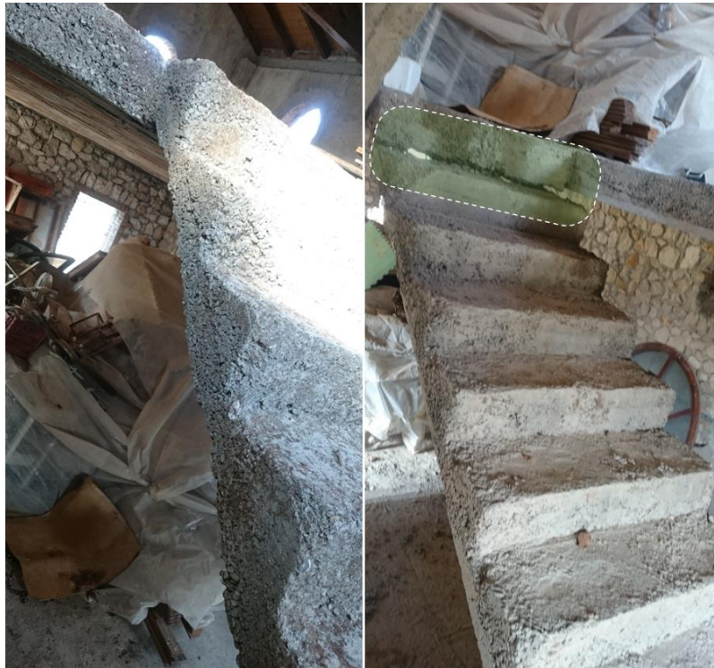
Figure 51: Very low quality of the material used in masonry building, support failure due to improper detailing
