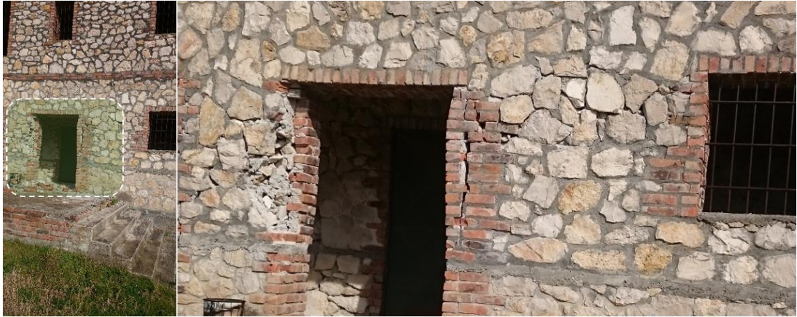
Figure 44: Disintegration in stone masonry building
