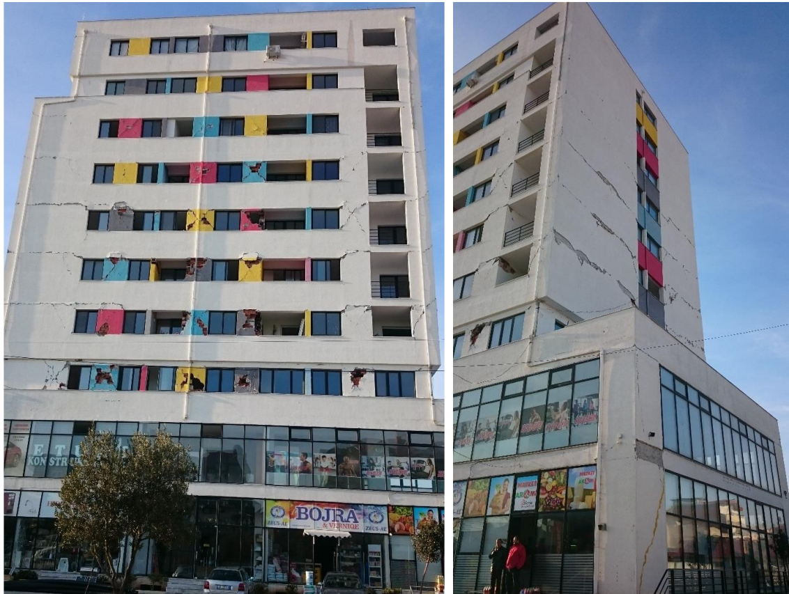
Figure 12: Heavily damaged high story Reinforced Concrete building
