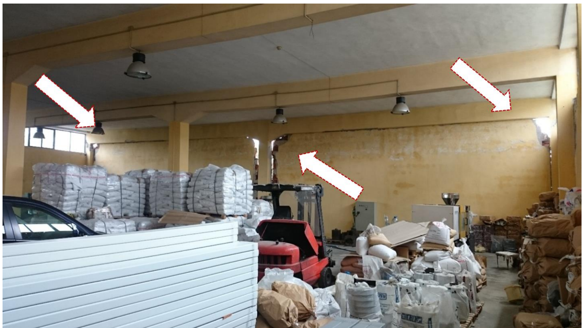
Figure 33: Out of plane failure of partition walls
