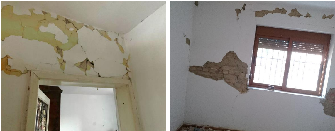
Figure 37: Spandrel crack above the openings (URM building)
