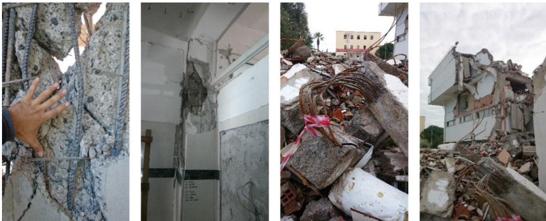
Figure 18: Inadequate detailing caused buckling of longitudinal reinforcement in plastic hinge regions (spacing of transverse reinforcement is indicated by thumb and index fingers as shown in the left)
