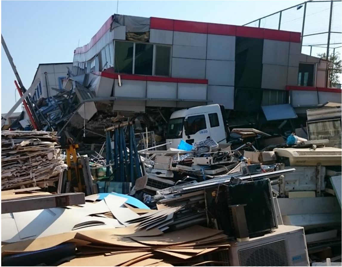
Figure 23: Reinforced concrete industrial building collapsed completely
