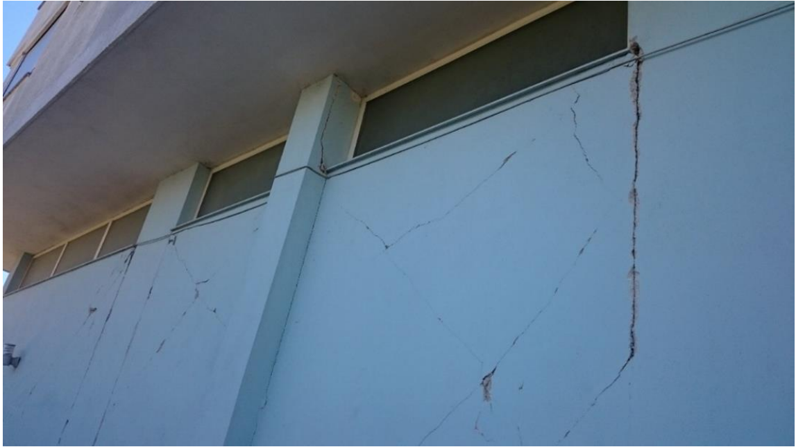
Figure 16: Short column formation and in plane failure of partition walls
