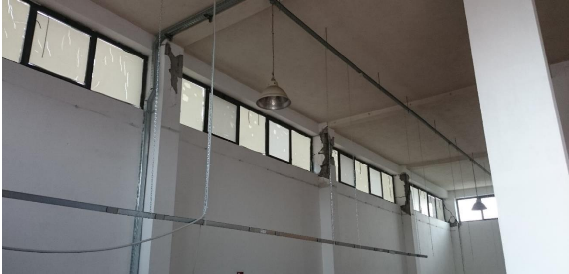
Figure 14: Formation of short column due to band window
