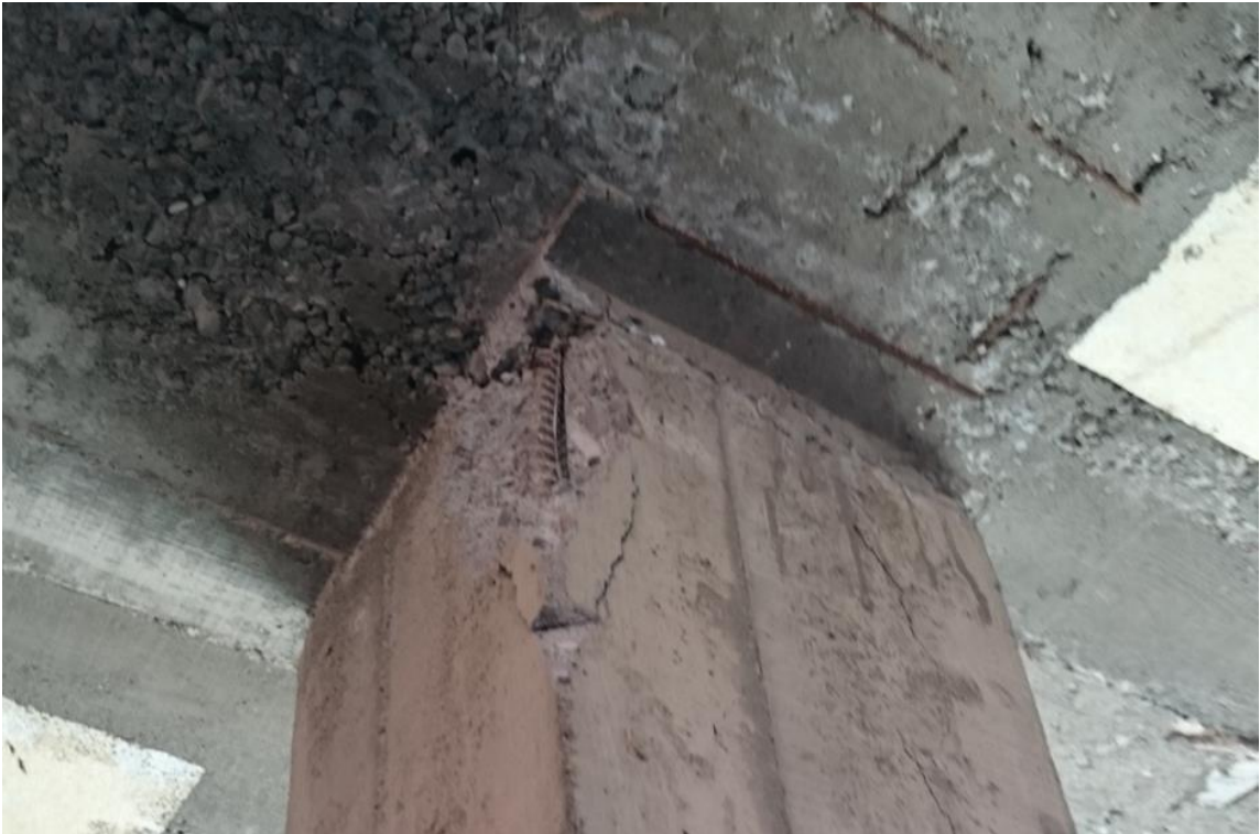
Figure 21: Insufficient stirrups, bar buckled
