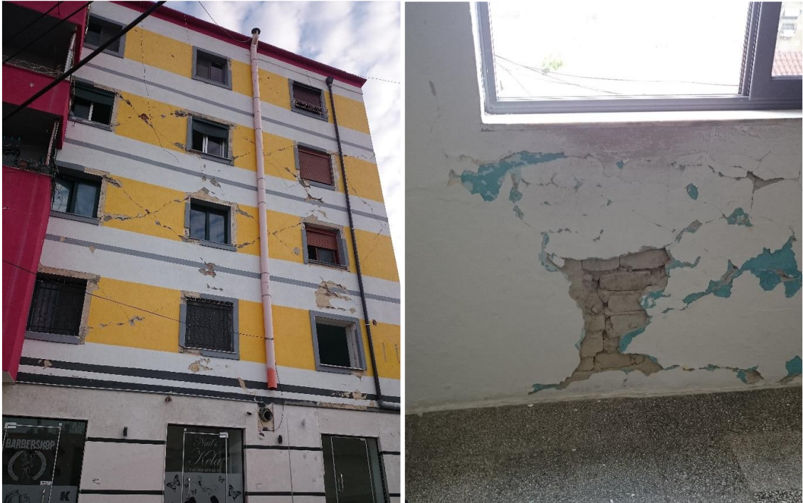
Figure 39: Shear cracks on the front façade of a masonry building
