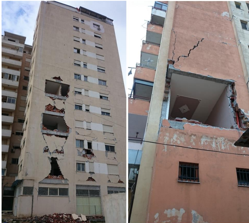
Figure 35: Heavily damaged high-rise RC building
