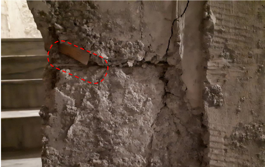
Figure 24: Poor quality of concrete, part of formwork found inside the concrete
