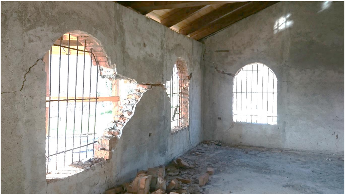
Figure 46: Heavily damaged pier of masonry building
