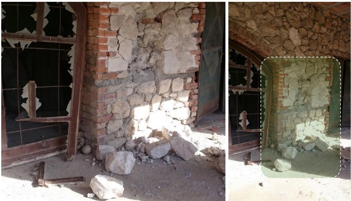
Figure 45: Pier damage on a stone masonry building
