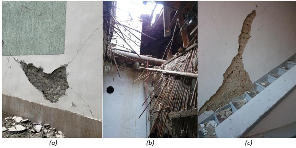
Figure 50: Damaged masonry buildings, a) spall of concrete cover of concrete from diagonal shear cracking, b) failure of the roof on adobe building, c) moderate damaged stair connection
