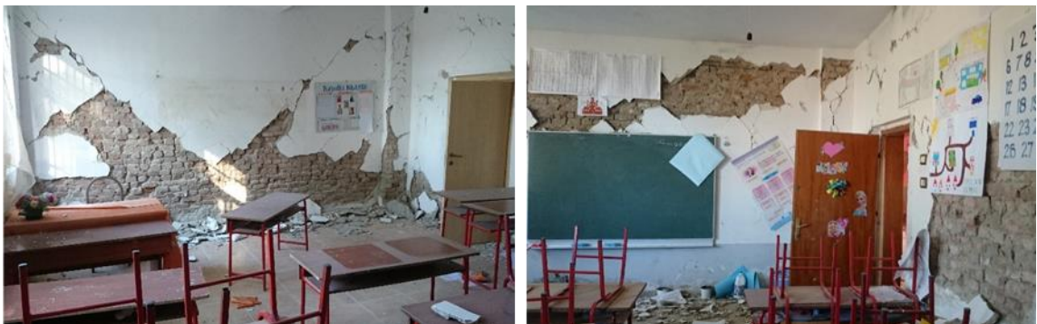
Figure 49: Poor material quality of a school damaged during November 26 earthquake
