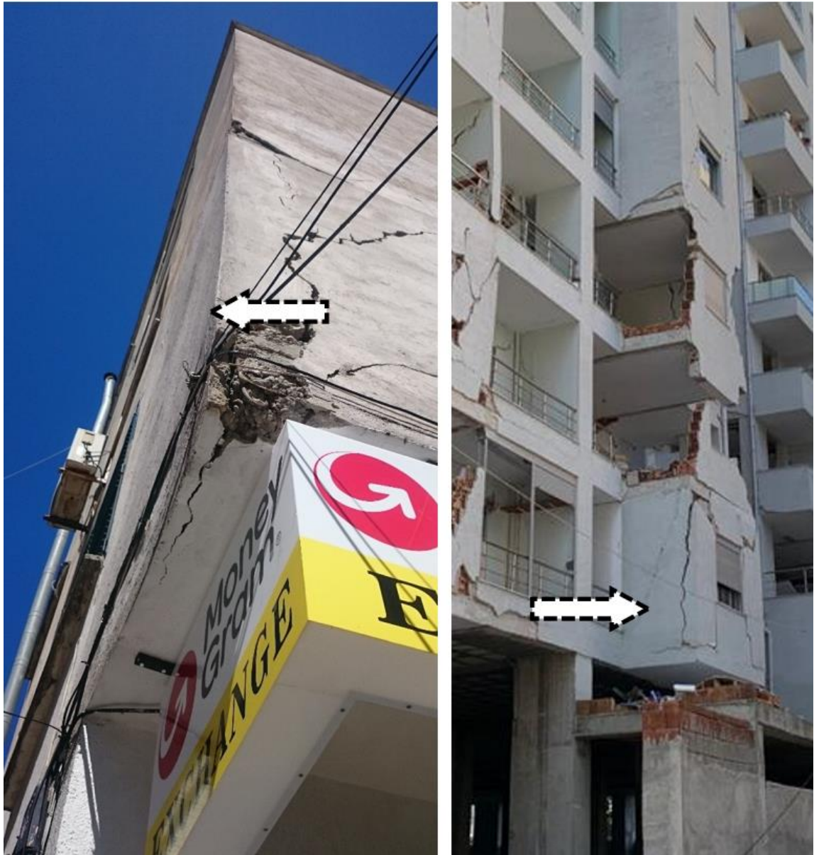
Figure 30: Heavy overhang and failure at the corner
