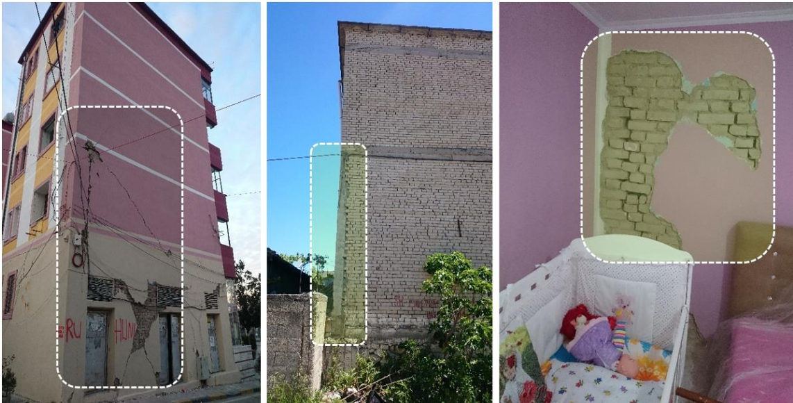
Figure 42: Example of residential URM buildings with cement mortar and RC floor and roof diaphragms: Formation of heavy shear cracks on the corners
