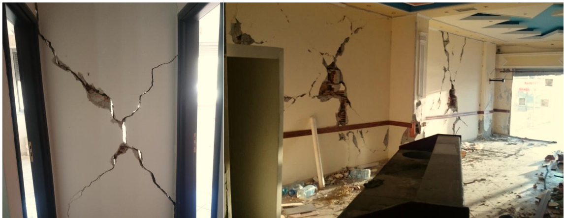
Figure 31: In-plane failure of partition walls
