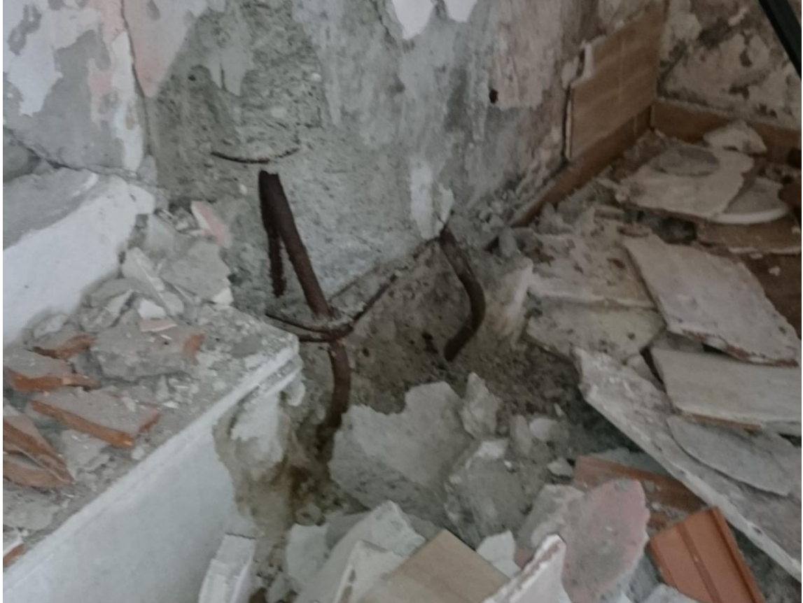
Figure 19: Buckled rebars on a reinforced concrete column base
