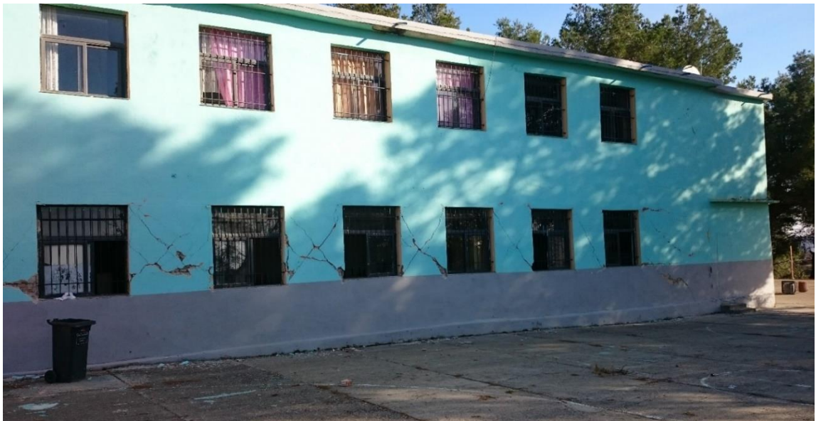
Figure 48: Shear crack on piers of a masonry school building
