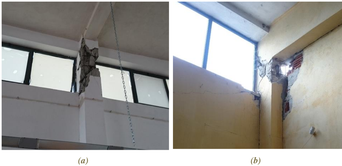
Figure 15: Typical shear failure of short columns in Reinforced Concrete buildings
