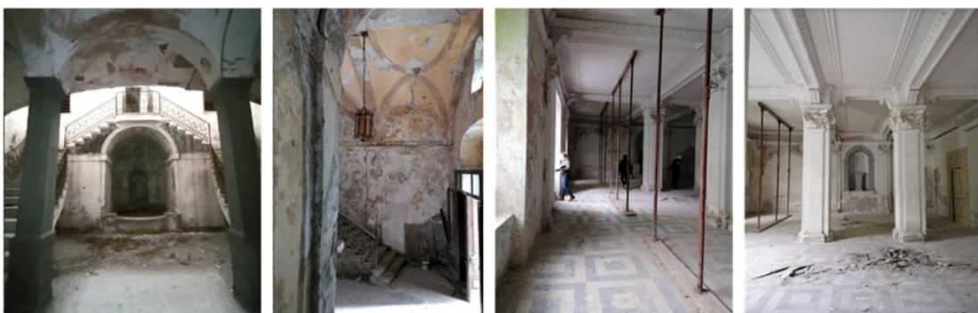
Figure 3. The condition of deterioration observed in the 'Edifici Mondo' is attributed to Mariarosaria Angrisano, Martina Bosone, and Antonia Gravagnuolo [18].
