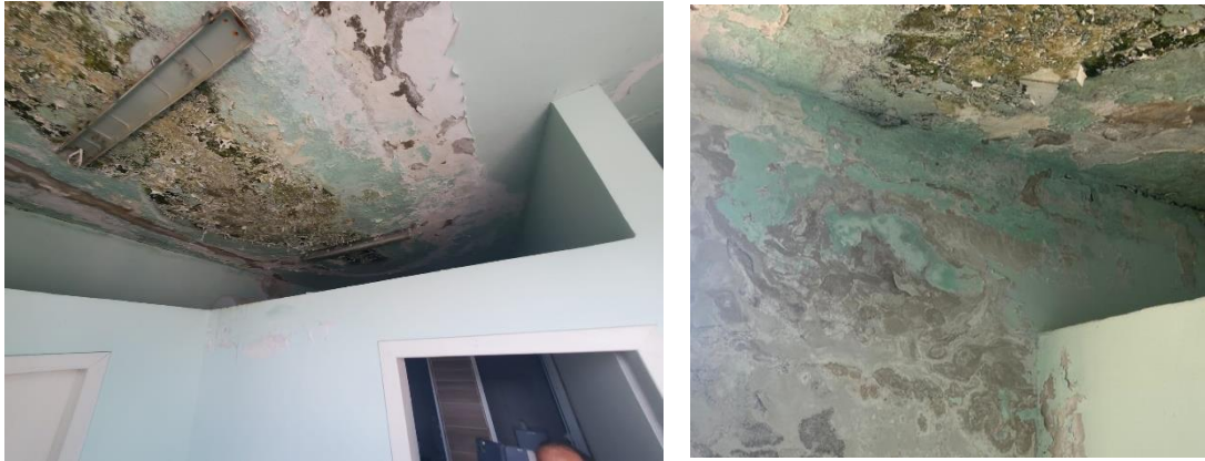
Figure 14. Damage to floor slabs and perimeter walls on the top floor due to the presence of moisture.
