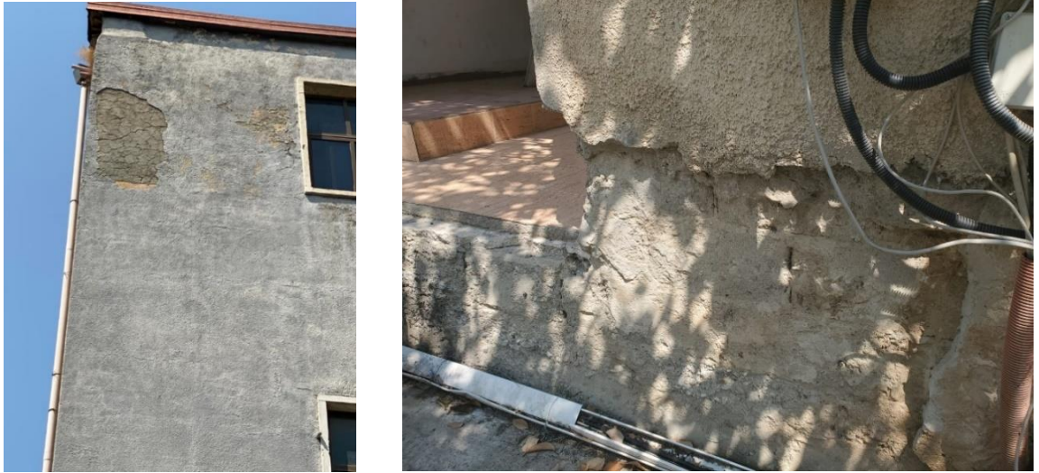
Figure 16. Damage to perimeter walls on the top and ground floor.
