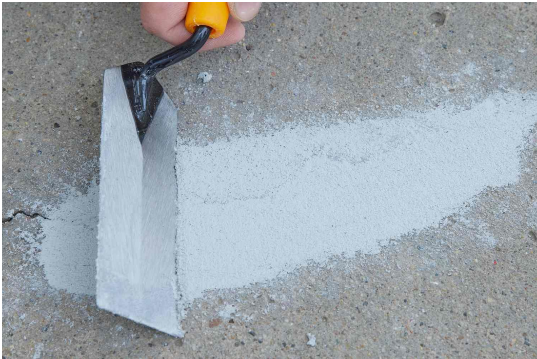
Figure 35. The cleaning and repair of existing surface cracks on the floor slab.
