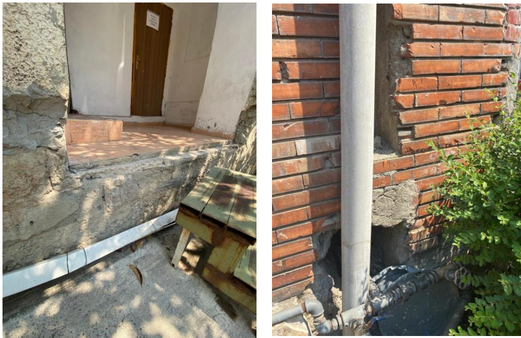
Figure 14. Observation of the masonry on the ground floor where concrete blocks are visible.
