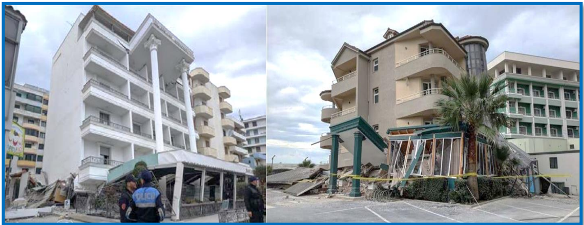
Figure 11. Collapsed buildings in Durrës, Albania due to the “soft storey” irregularity (McKenney, 2019)
