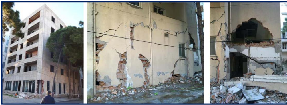
Figure 12. Damage to RC building in Durrës, Albania due to torsional effects: a) a view of the building after the earthquake; b) damaged masonry infill at the ground floor level (adjacent to the staircase) and c) damaged staircase area
