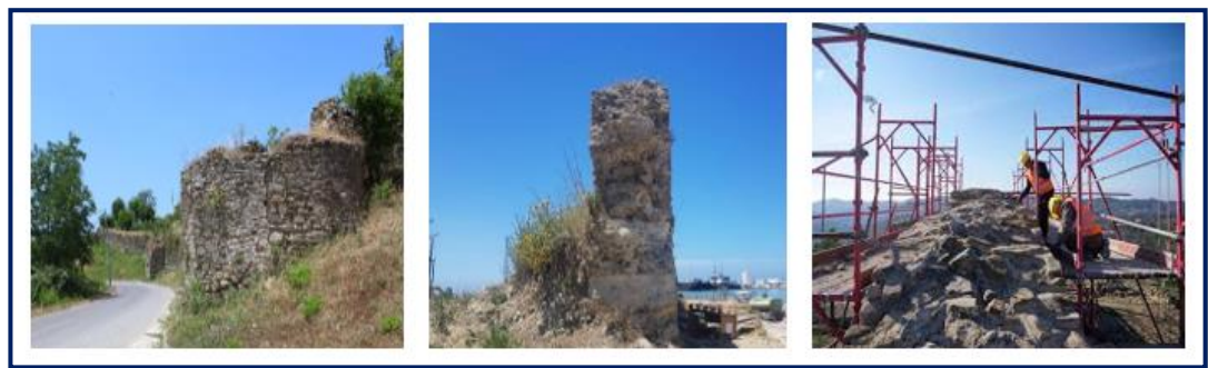
Figure 7. Gate walls at Porto Romano; (a) the wall before earthquake , (b) the gate wall damaged (c) the wall under reconstruction
