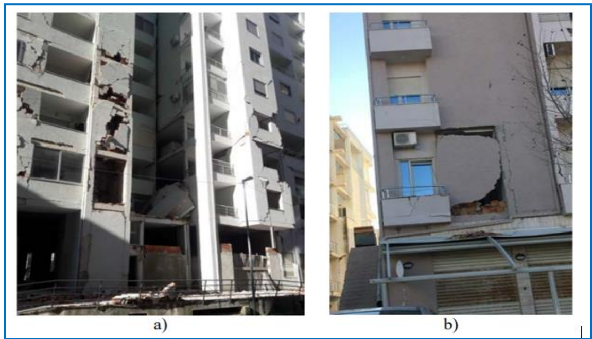
Figure 14. Severe damage and failure of masonry infills in RC frame buildings in Durrës, Albania due to the November 2019 earthquake
