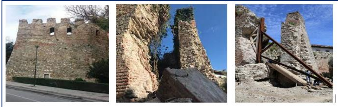
Figure 6. Durrës Castle-Tower 'C' and fortification walls (a)before earthquake , (b) collapse wall , (c) the structure of steel reinforced
