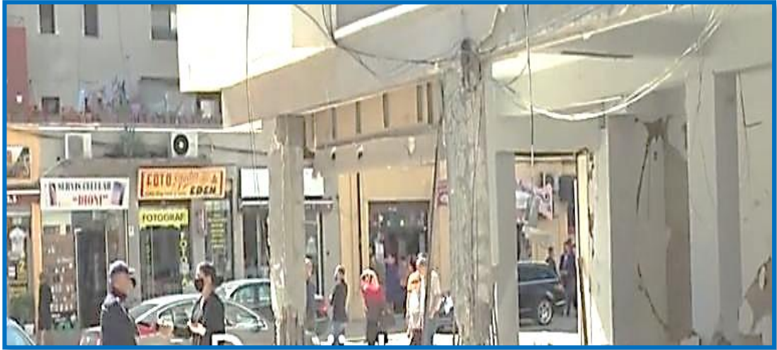
Figure 19. Damages made in the building by the earthquake
