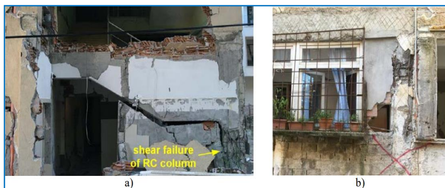
Figure 13. Damage of RC buildings due to the "short column" effect in the November 2019 Albania earthquake: a) impact of the stair support on supporting columns and b) impact of partial masonry infill due to the openings
