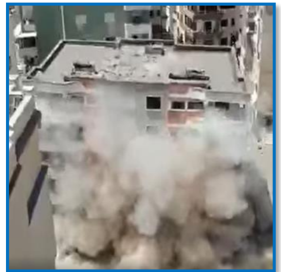
Figure 18. Vip building collapse
