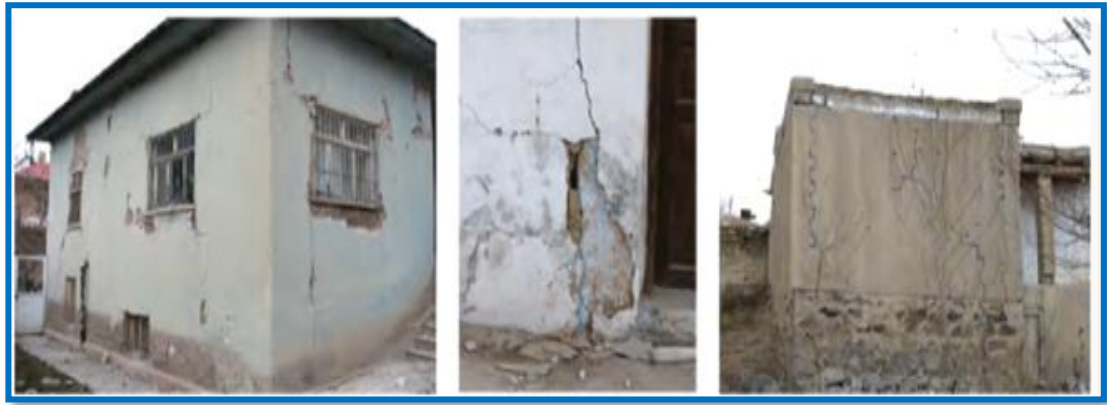
Figure 3. Unreinforced brick building with damage
