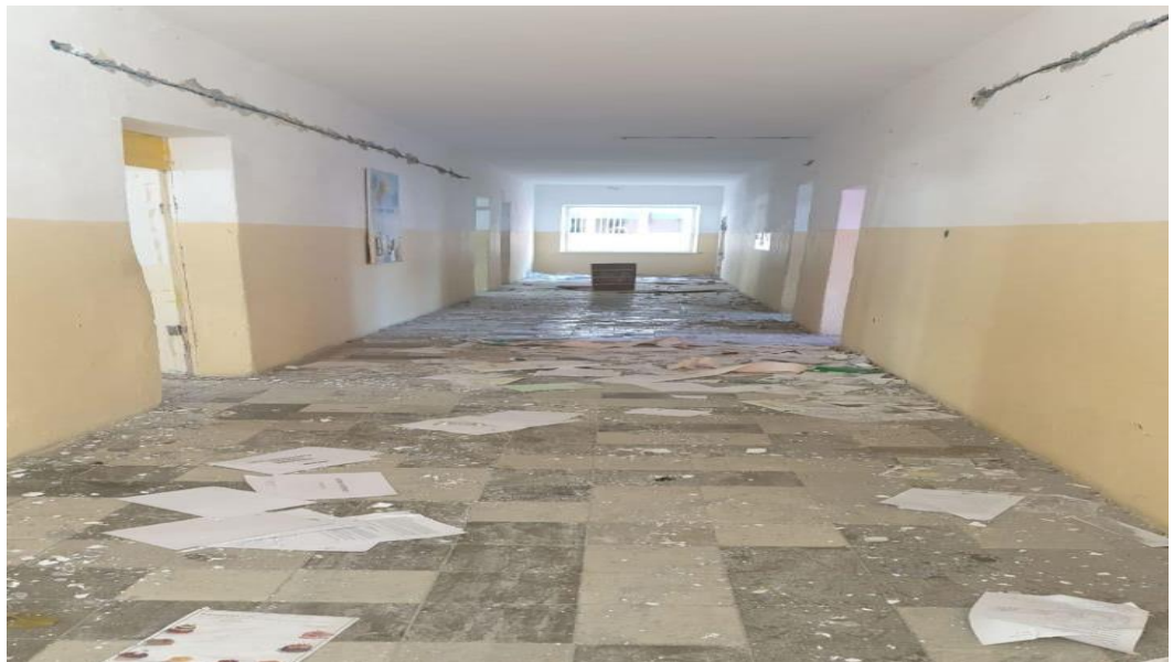
Sliding shear failure of masonry
