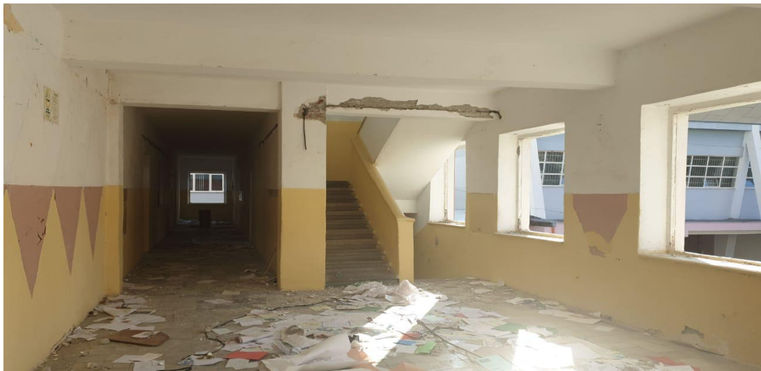
Sliding shear failure of masonry
