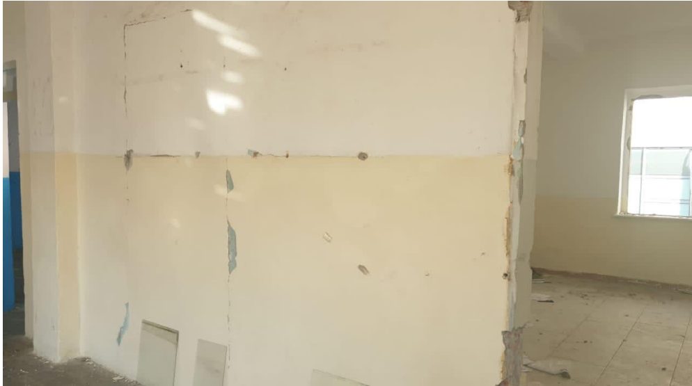
Non structural damages in masonry
