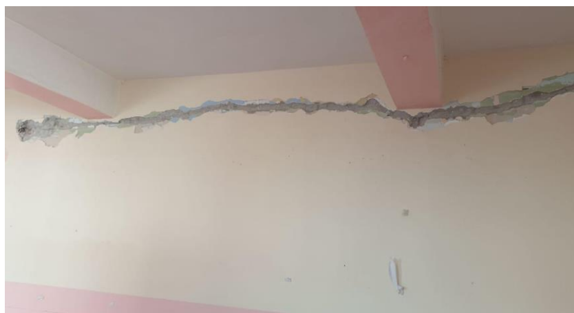
Shear sliding failure of masonry
