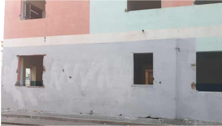
Diagonal cracks on masonry
