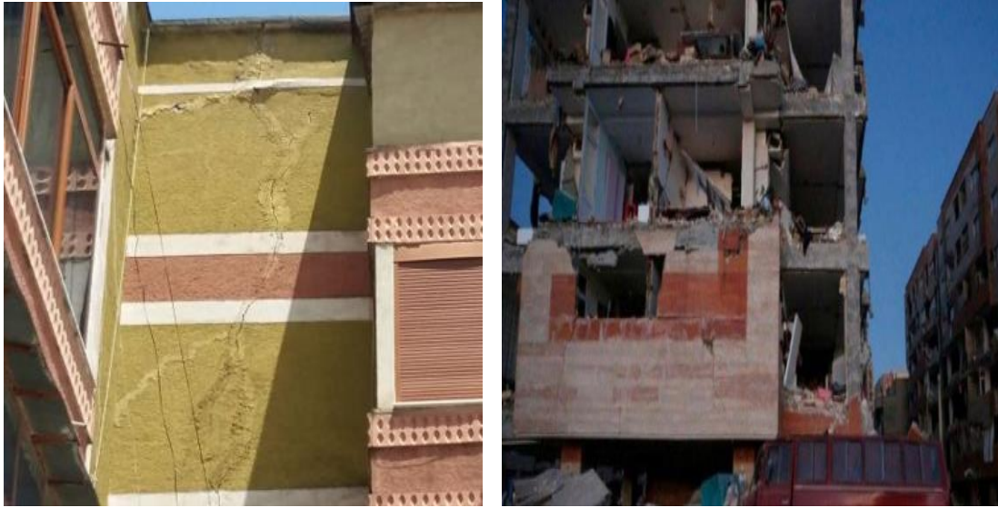
Fig 59. Albanian buildings damaged during earthquake disasters in Elbasan. Many buildings designed according to old designing codes, with no good reinforcement design for shear.
