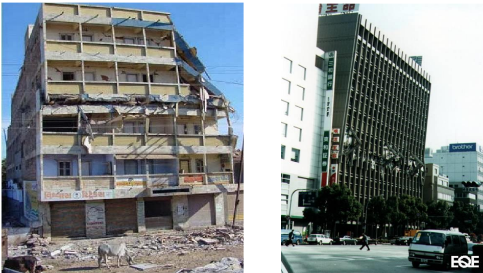
Figure 11. Collapse of intermediate story in a 6 storey RC frame commercial building in Bhuj. Figure.12. Mid-story collapse, Kobe earthquake.
