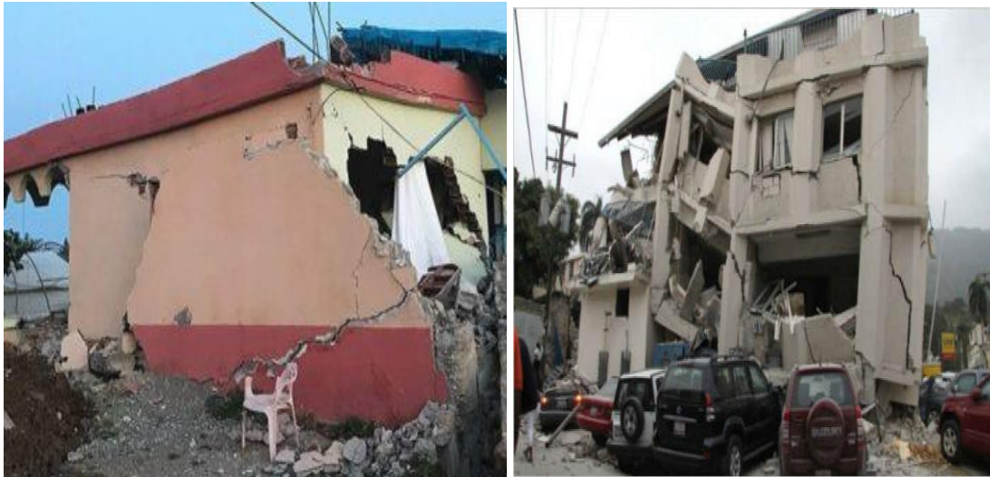
Fig 57. Building collapse due to an earthquake of 5.1 magnitude in Bulqize, 2018. Building are lack of shear walls and they also are constructed with no proper structural design.
