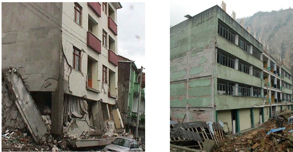
Figure 9. Soft story failure in an Izmit apartment building. Figure . Reinforced concrete framed structure, masonry infill with soft story failure at the bottom level. [Pathmanathan Brabhaharan, 2012]
