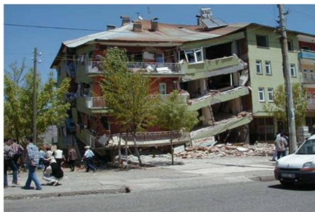
Figure 41. Collapse of adjacent buildings during the Bingöl earthquake.2003.
