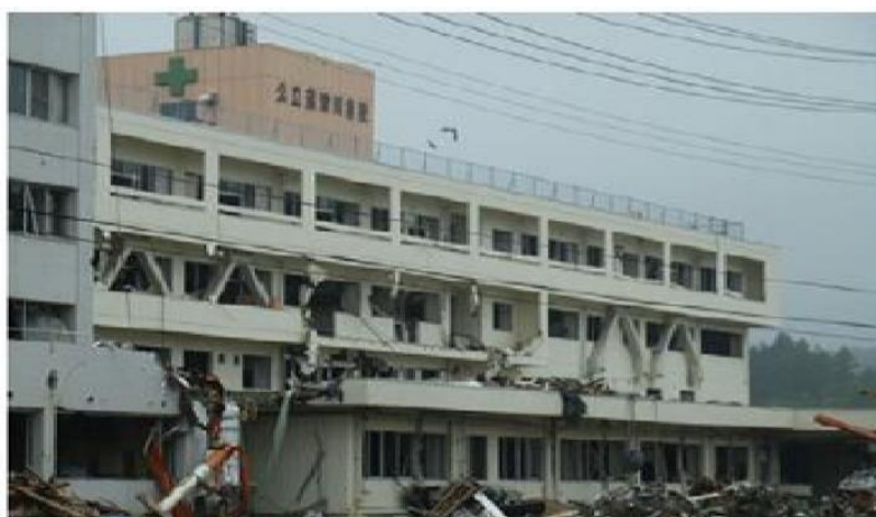
Figure 36. Failure of balconies at Shizugawa Hospital during Tsunami 2011 [Fraser et al. 2013]
