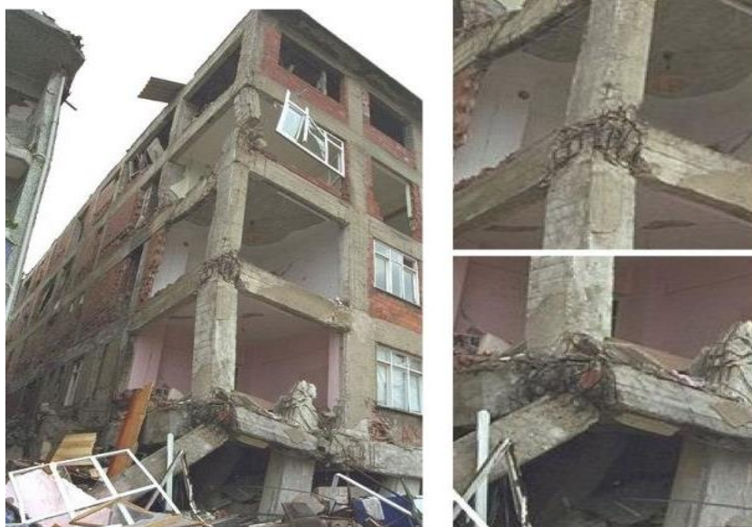
Figure 48. Partial Building Collapse due to failure of beam-column joints in the Izmit, Turkey earthquake of August 17, 1999.
