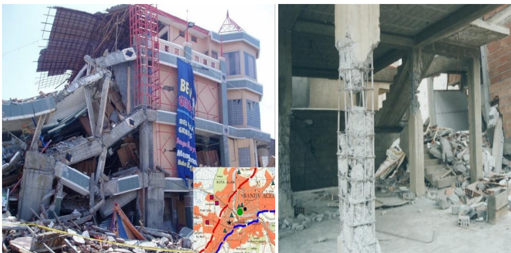
Figure 50(left).Pante Pirak Supermarket, a 3-story building, the collapse was due to poor quality of construction, and right, Seismic deficiencies - very poor quality of concrete (2003 Boumerdes earthquake)
