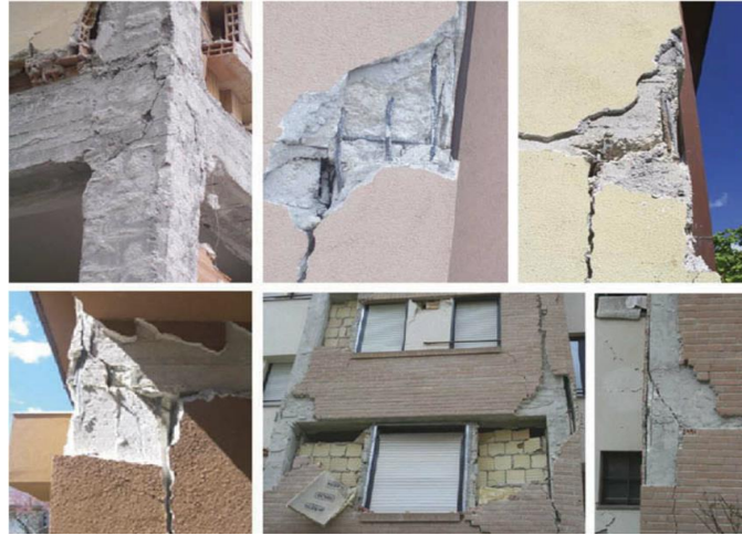
Figure 23. Corner beam-column joint failure during the Abruzzo earthquake [ReLUIS, 2009]
