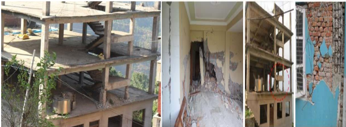
Figure. 30 RC frame building under short column effect. (Vahidi 2009) Figure 31. Examples of short-column failure due to the presence of (A) staircase landing and infill, (B) staircase landing beam, and (C) infill panels with openings. [H.Varum 2015 Nepal]
