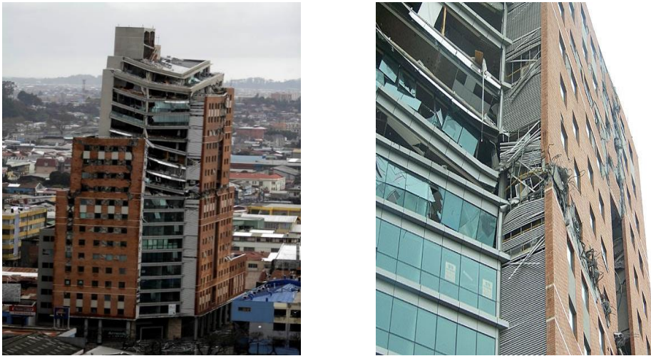
Figure 20. Torre O'Hings high rised building., built in 2007 and consisiting in many structural setbacks along the building height. The earthquake damage included partial collapse at three levels above mid-height.
