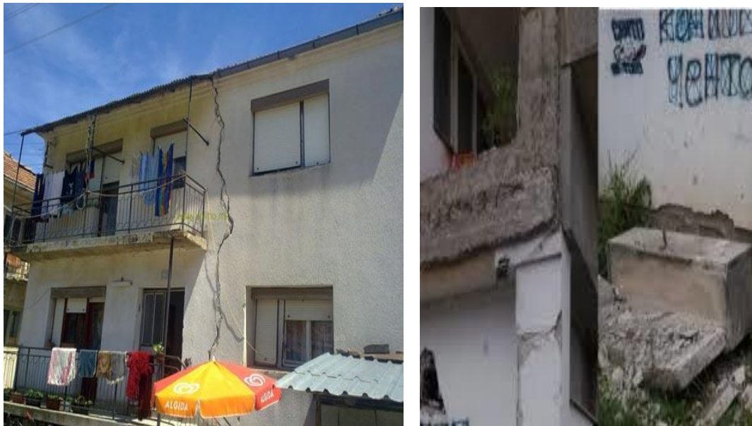
Fig 56. Building damages during an earthquake of 4.5 magnitude in Oher, 2012 due to non-ductility of structure and poor materials quality.
