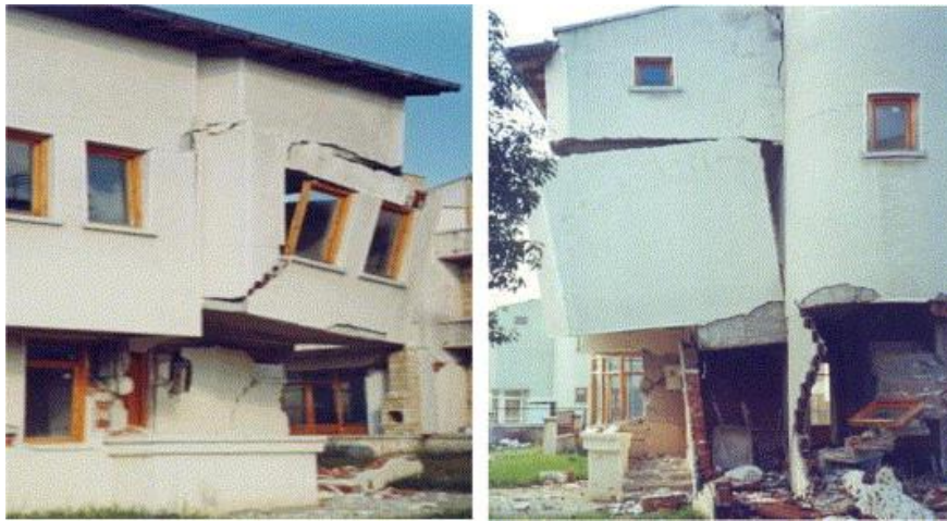
Figure 35. Earthquake failures of cantilever projections buildings in Turkey. [M.Dogan 2007]
