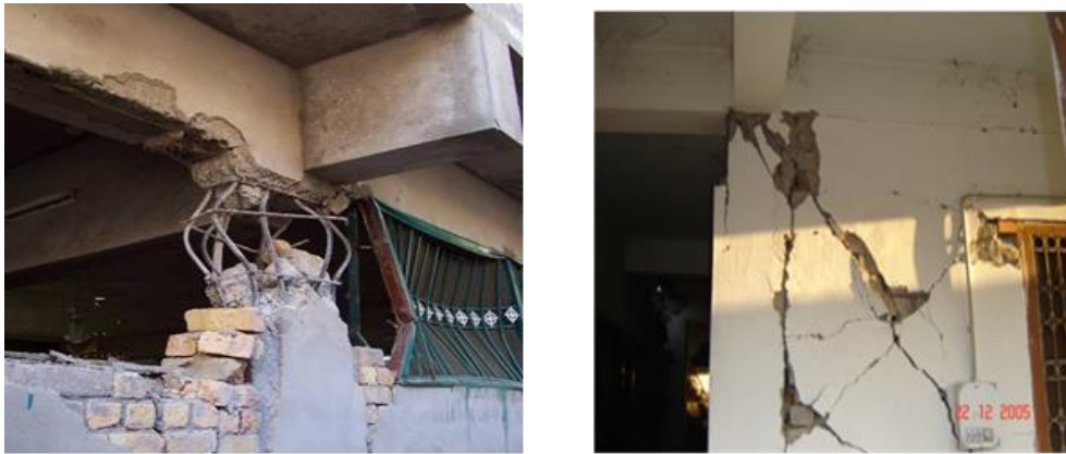
Figure 33. Short column due to partial height infill wall [WHE Report, Nepal]
