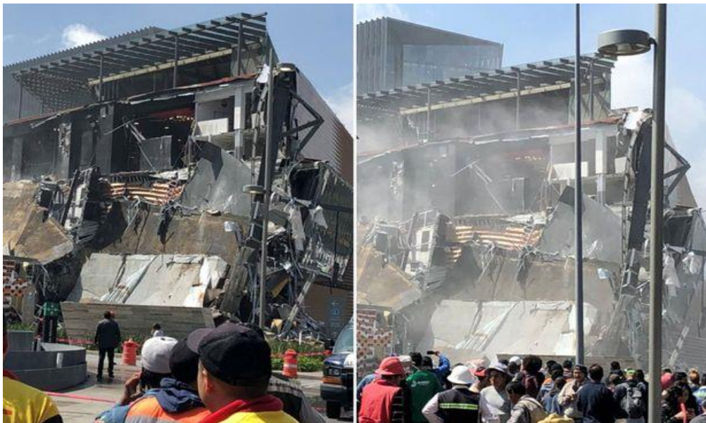
Figure 15. Brand new shopping centre in Mexico collapses under weight of heavy roof garden. [News Locker, 2018]
