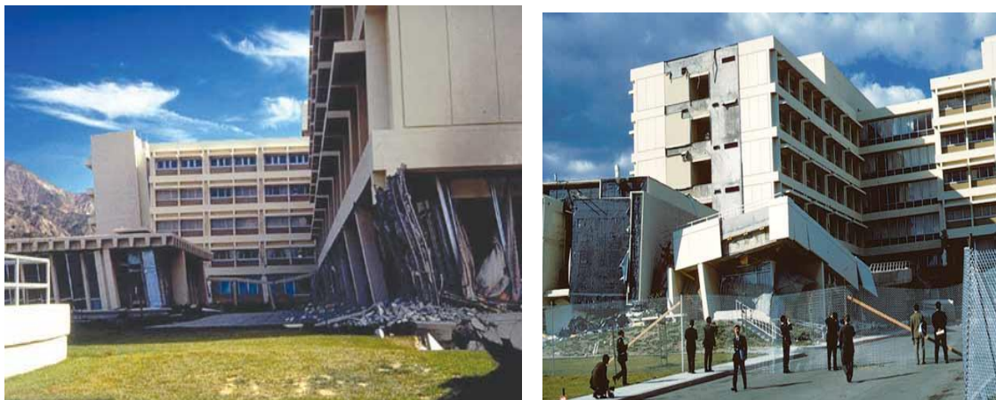
Figure 17. First floor collapse of the main buildings of the Olive View Hospital [by L. Hashizume, E. Loh]
