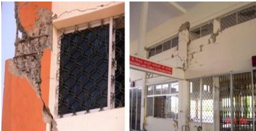
Figure 34. Shear failure due to short column effect observed in Port-Blair, India, during Sumatra earthquake 2004.
