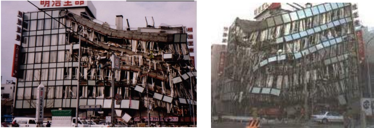
Figure 7. Partial collapse of a 6-story commercial building (Chou Ward) with a torsional irregularity. [Photo courtesy of Charlie Kircher]
