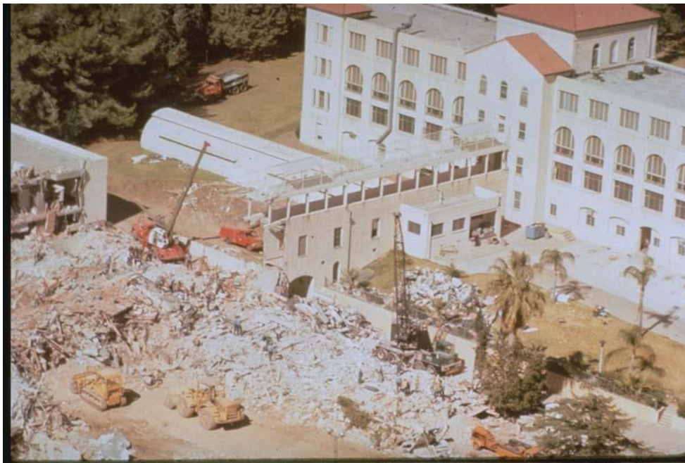
Figure 52. Example of non-ductile concrete frame building collapse at the Veterans Administration (VA) complex in the 1971 San Fernando earthquake.
