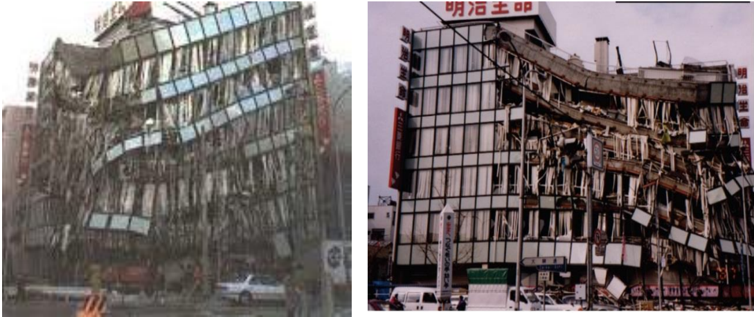
Fig 54. Partial collapse of a 6-story commercial building (Chou Ward) with a torsional irregularity.
