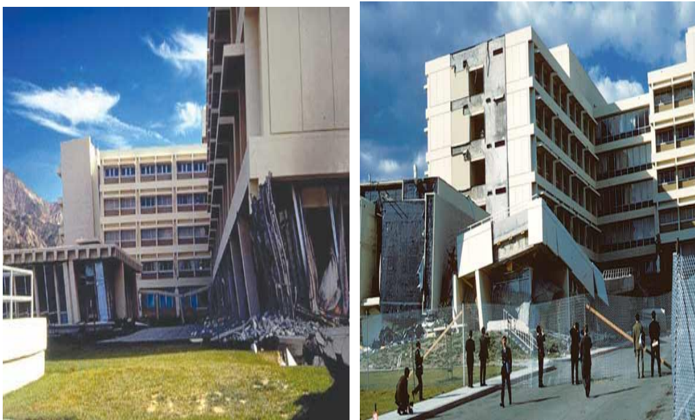
Fig 53. Damage and collapse of buildings of the Olive View Hospital and Sylmar hospital due to the 1971 San Fernando earthquake.
