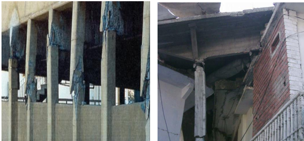
Figure 24. Damaged parking structure Whittier Narrows (Los Angeles) earthquake, 1987 The deep spandrels create a strong-beam, weak column condition.
