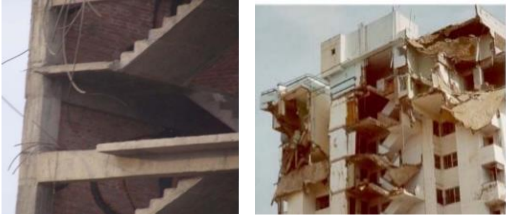
Figure 32. Short column effect due to staircase landing beam. [Binay Shrestha, 2015]
