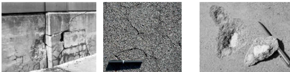
Figure 1. a) Expansion, b) Cracking, c) Popouts
