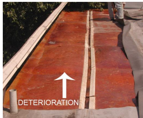
Figure 9: A building failure on thermal insulation panels on roof flooring (Güzelçoban, 2007)
