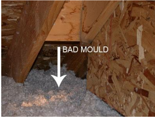
Figure 12: Bad mold growth on insulation materials in a cold roof (Güzelçoban, 2007)
