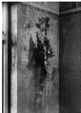
Figure 3: Bad mould growth on exterior walls interior surfaces (Ransom, 2005)
